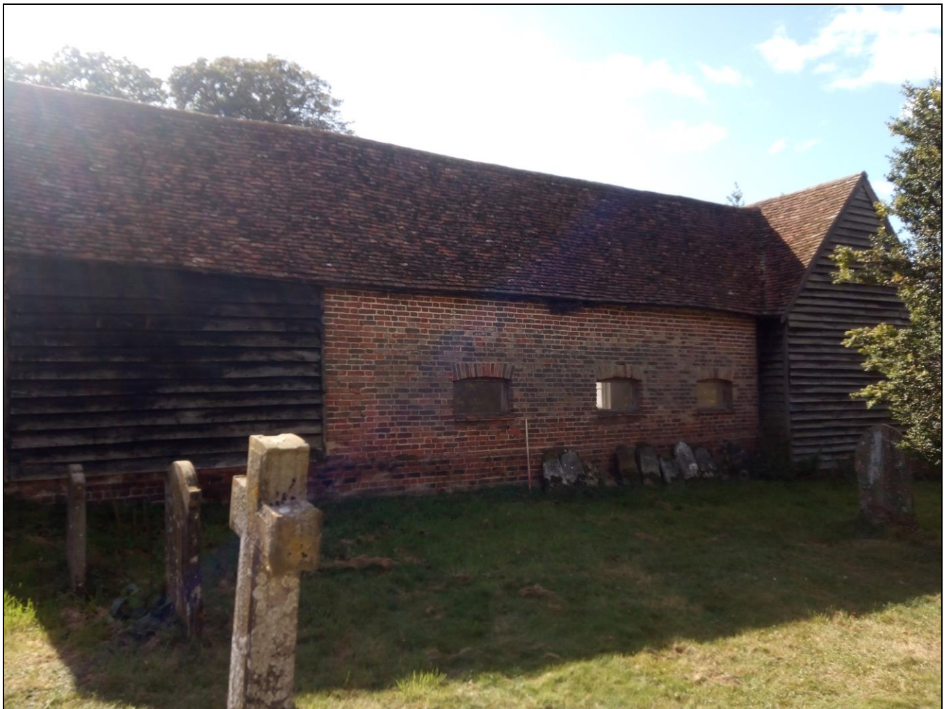
Figure 22. The north west wall of the coach house was facing the cemetery. The central part of this wall showed signs of having been re-built.
