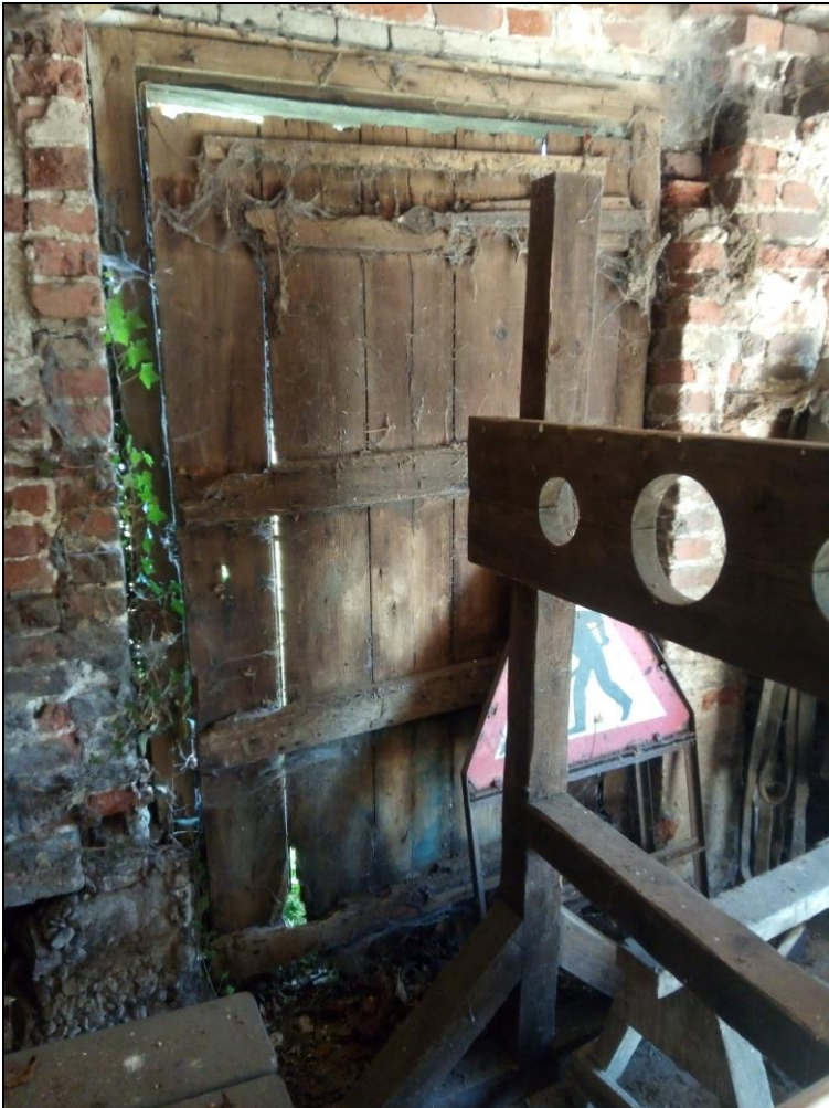
Figure 18. The original entrance to the dovecote with its old wooden door. North east facing photo.
