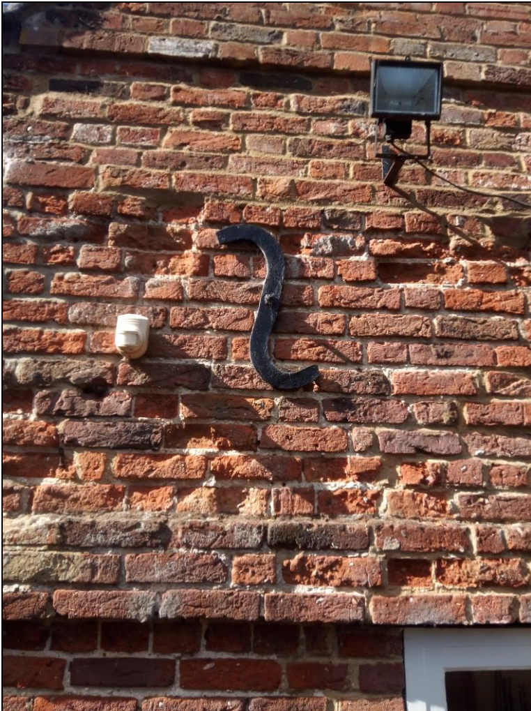
Figure 21. S-shaped iron reinforcement in the north east wall of the coach house.
