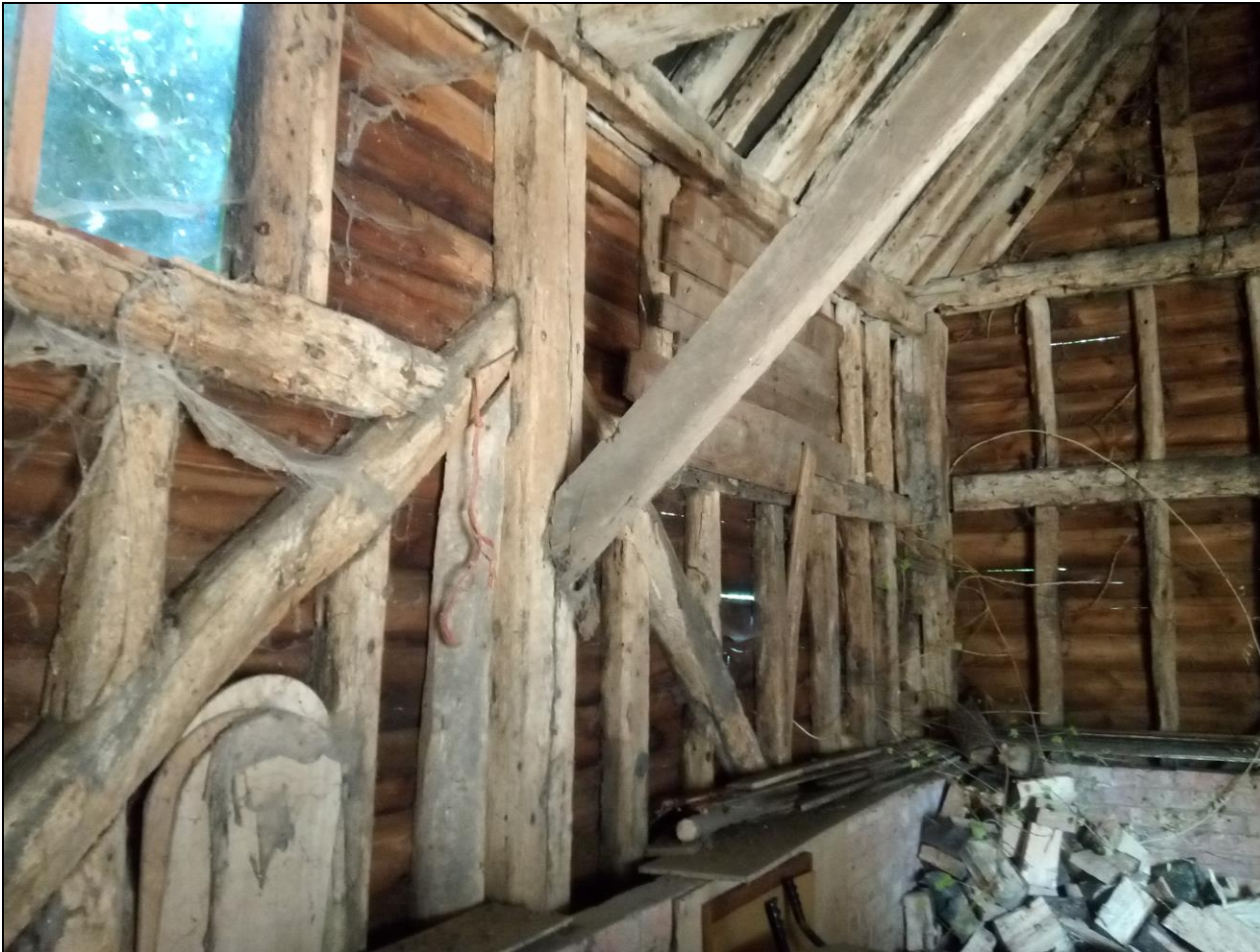
Figure 30. The joints between the roof and wall beams in the wooden outbuilding next to the coach house is likely to be of 17 th century date. West facing photo.
