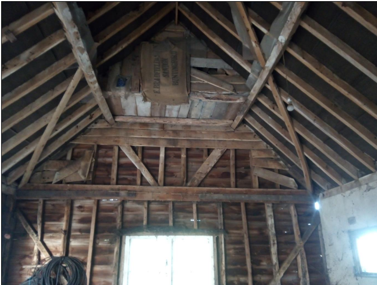
Figure 27. The wooden beams in the supporting structure of the old outhouses consisted of a mix of old and younger timber. South east facing photo.
