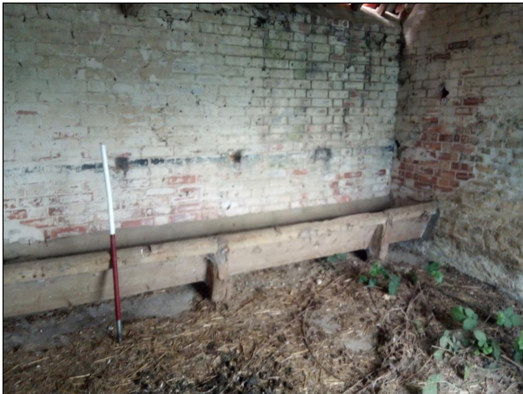
Figure 29. In the western part of the brick animal shed the wooden feeding rack was still intact. Photo from northeast.
