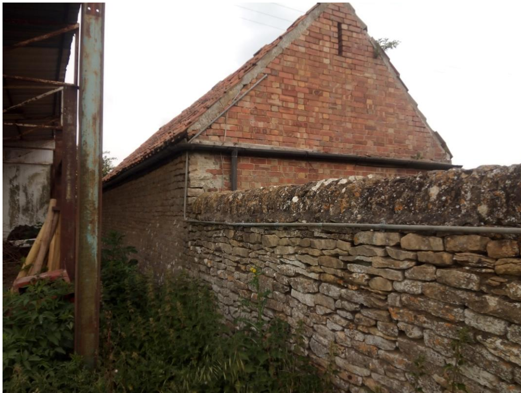
Figure 13. The old enclosure wall continued into the brick building in the southern part of the site. This suggests that the brick structure is of a later date.
