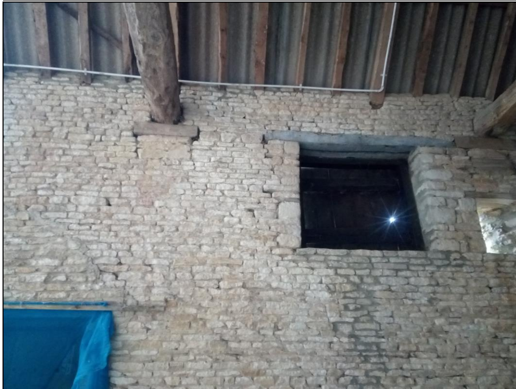
Figure 24. The wooden trusses of the 19 th century barn had at some point been replaced, or at least moved upwards by ca 0.5m, as the blocked up original beam slots were visible throughout the barn. Photo from south.
