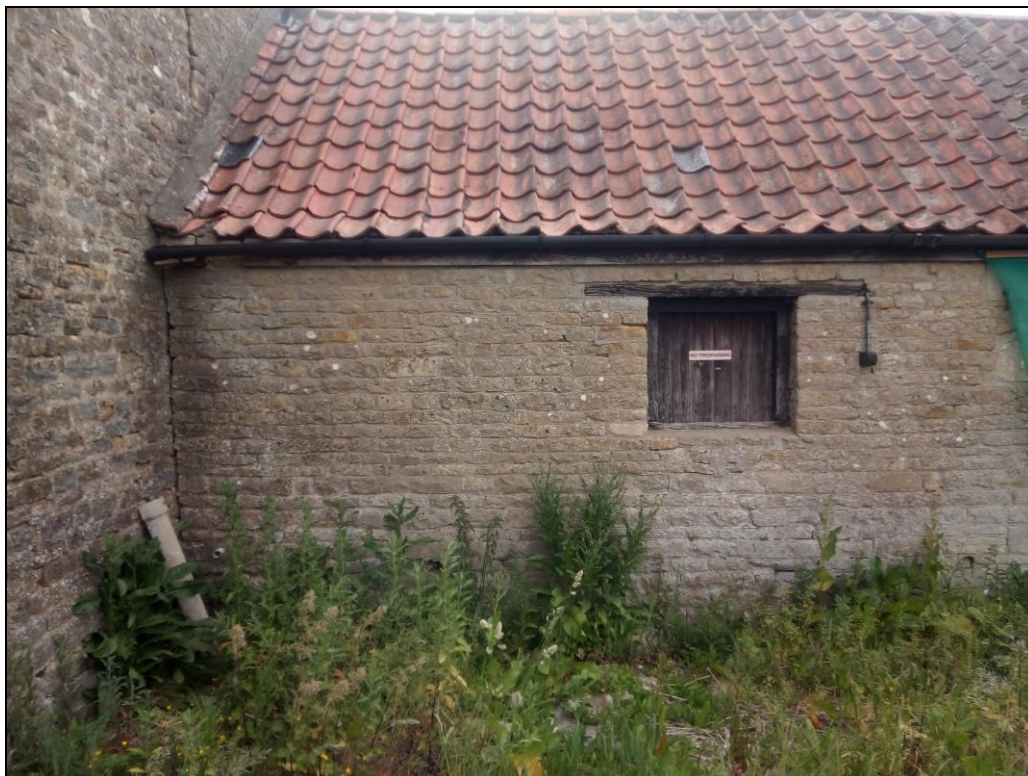
Figure 15. This stone extension of the original barn was possibly built during the later part of the 19 th century. Photo from west.
