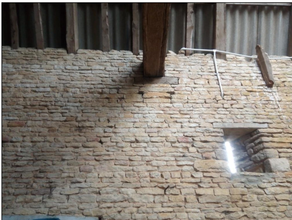
Figure 25. Another blocked up original beam slot in the 19 th century barn. Photo from north.
