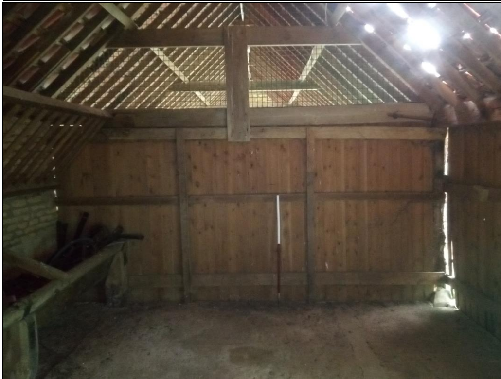
Figure 34. Interior of the partly wooden animal shed along the eastern enclosure wall. Photo from north.
