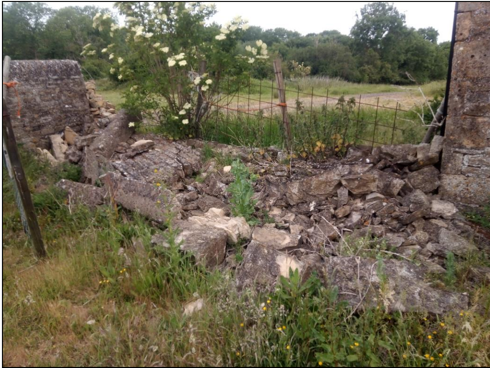
Figure 18. A part of the old stone enclosure wall had collapsed in the north west corner of the site. Photo from south east.
