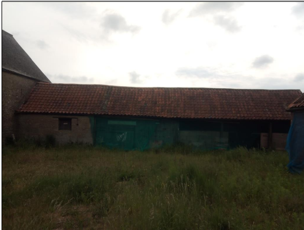
Figure 16. A partly wooden animal shed had been preserved along the original enclosure wall. The structure likely dates from before the year 1900. Photo from west.
