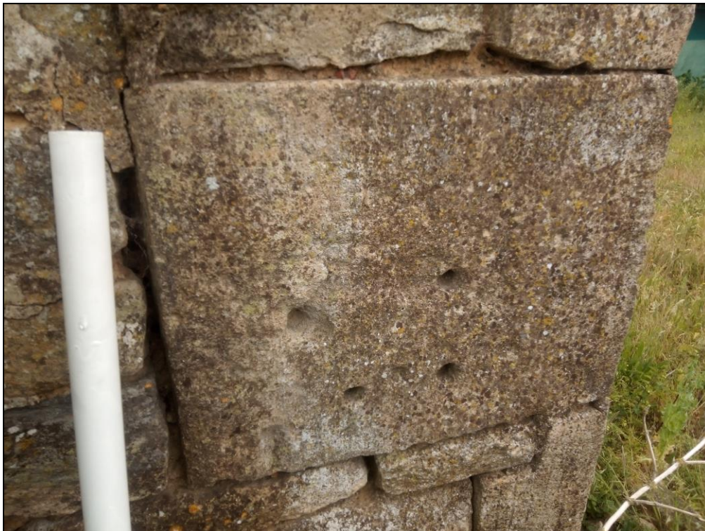
Figure 19. The original barn from the 19 th century contained a few re-used stones. This particular stone could be from an older church or farm building in the area. Photo from west.
