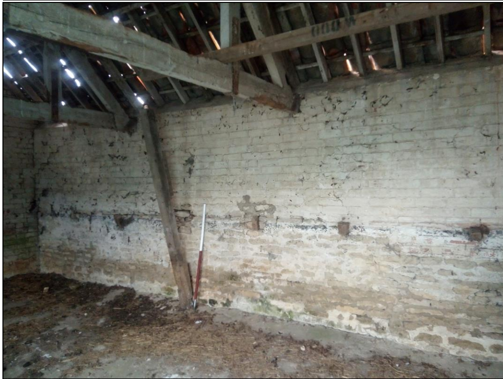
Figure 28. A wooden feeding rack had once been located along the southern wall of the brick animal shed, but its beam had been cut at some point. Photo from northwest.
