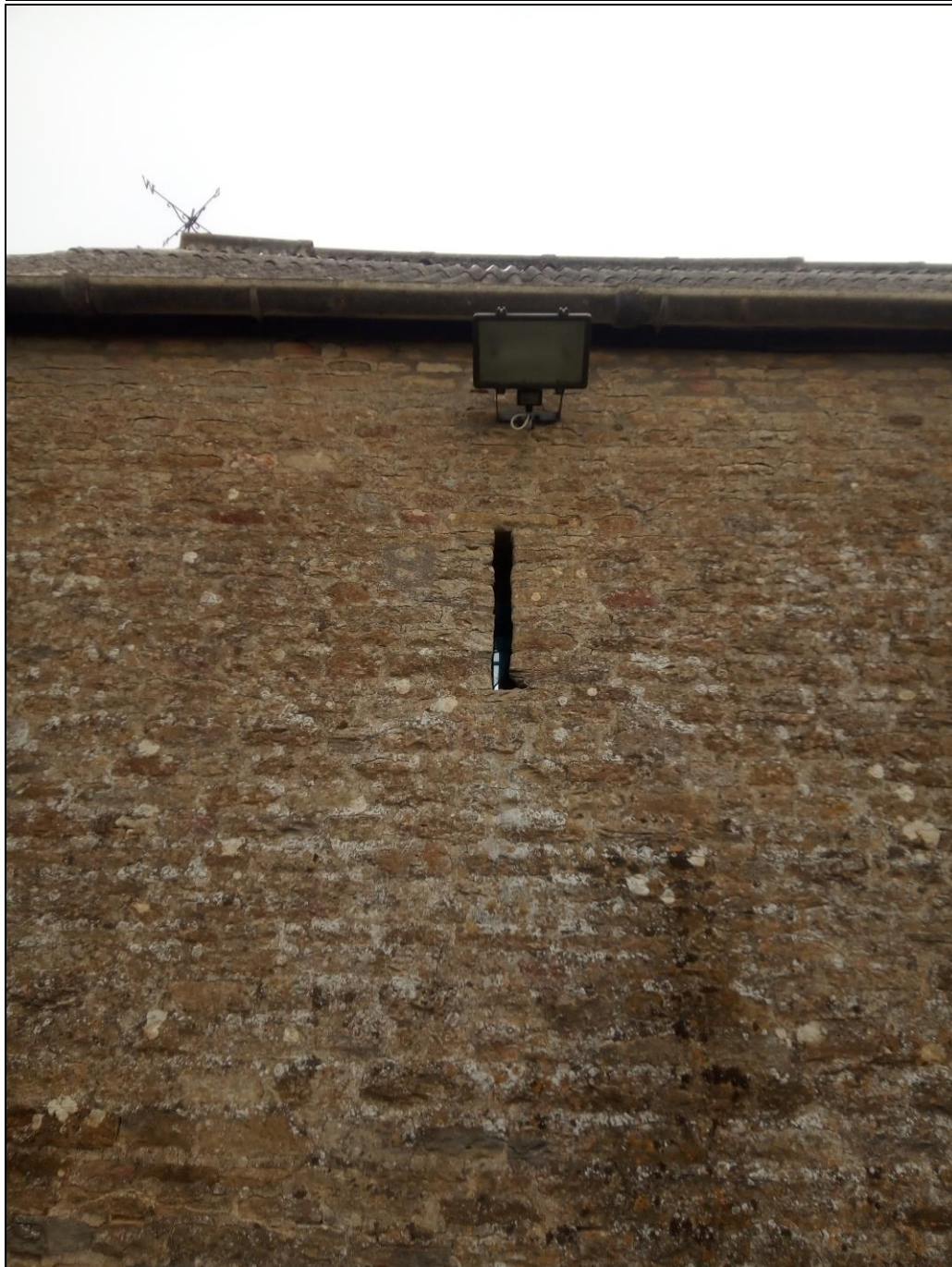
Figure 21. The narrow ventilation windows in the 19 th century barn are based on a much older design, and almost reminds of arrow slits in medieval castles. Photo from south.
