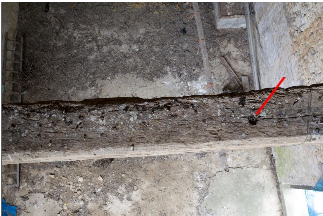
Drone photos from inside the main barn. Holes were identified on the upper sides of the wooden trusses, indicating that the beams may have been re-used in the barn.
