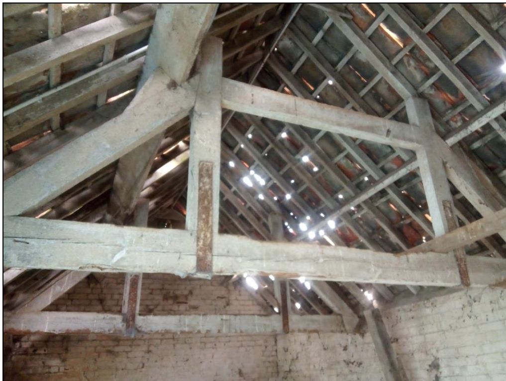
Figure 31. The wooden beams in the roof construction of the brick animal shed. Photo from west.
