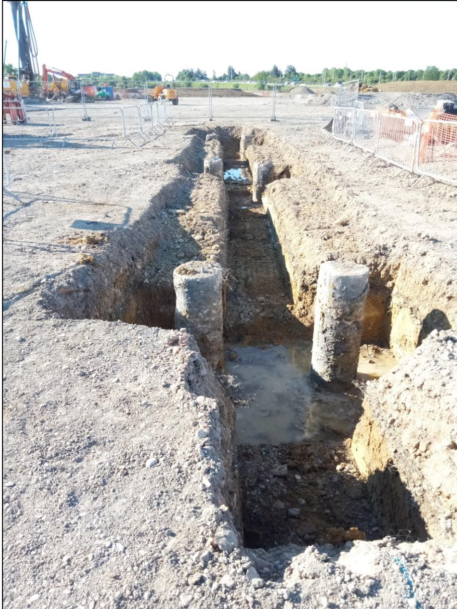
Figure 11. Digging the trenches for the new foundations between the concrete piles that had already been driven into the ground in some areas of the site. South facing photo.
