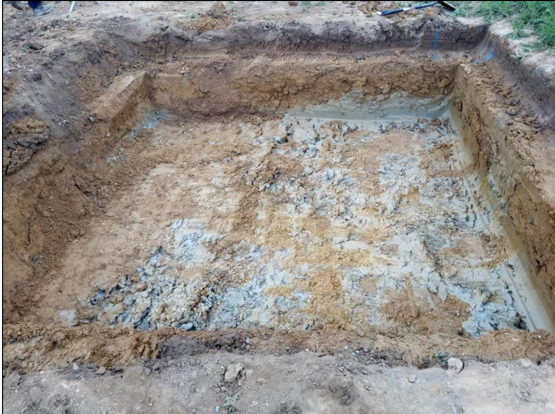
Figure 8. A quadratric trench for a new electrical substation in the eastern parts of the site. North facing photo.
