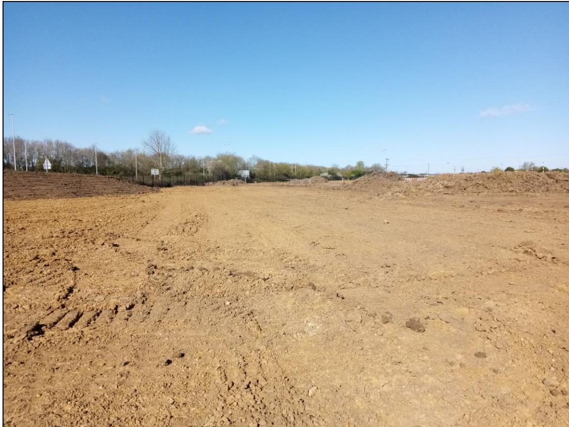
Figure 4. Overview of the southern part of the development area along A47. West facing photo.
