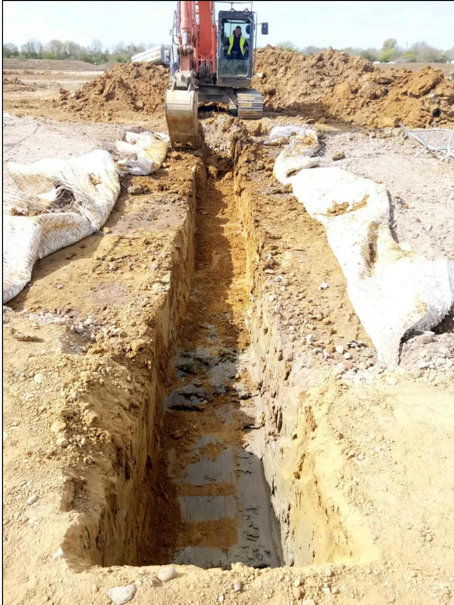
Figure 6. Example of a trench for drainage pipes in the northern parts of the site. West facing photo.
