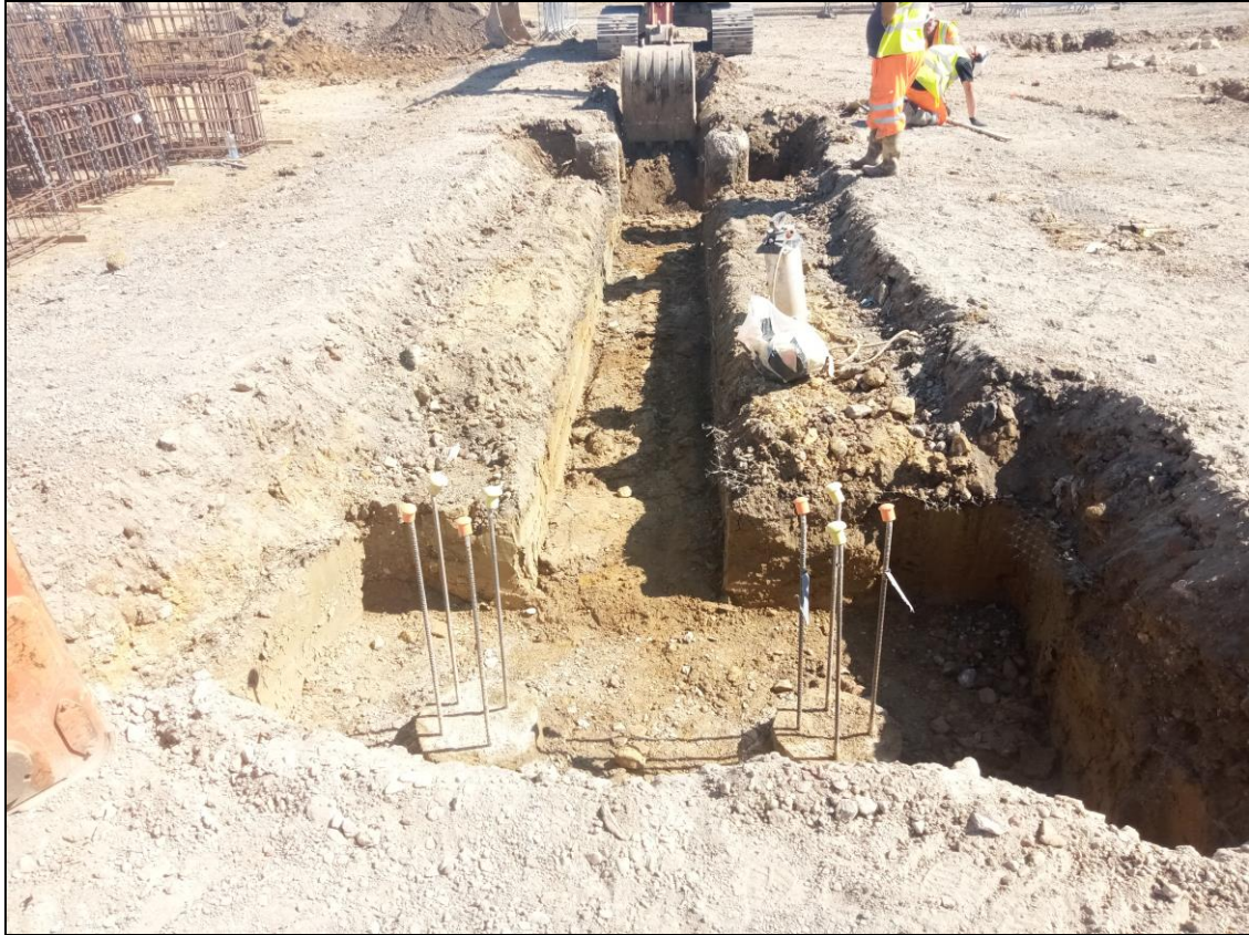
Figure 10. Digging the trenches for the new foundations between the concrete piles that had already been driven into the ground in some areas of the site. East facing photo.
