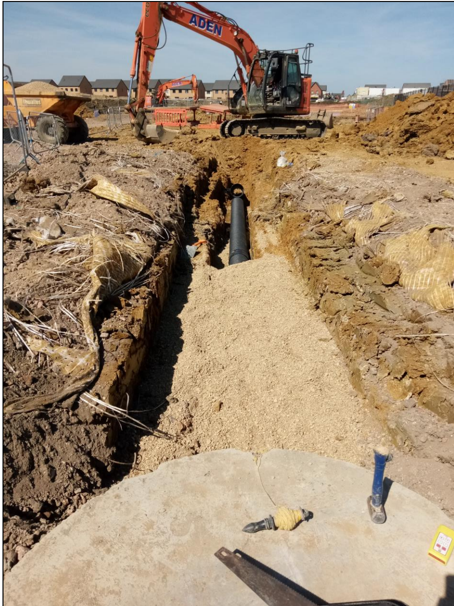
Figure 7. A drainage pipe has been put into a trench, and the trench is being backfilled with shingle. North west facing photo.
