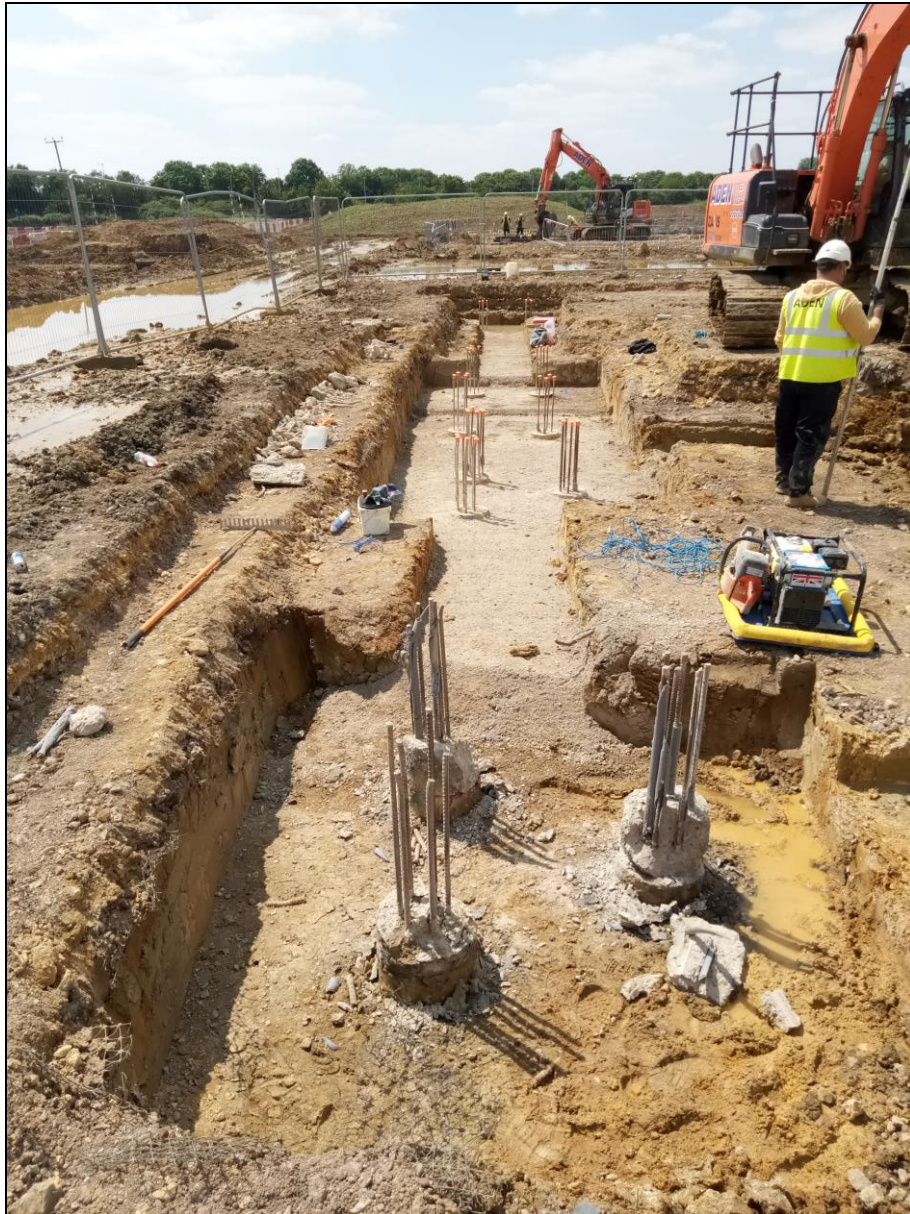
Figure 13. The concrete was being added between the existing piles to create a stable foundation for the new school building. West facing photo.
