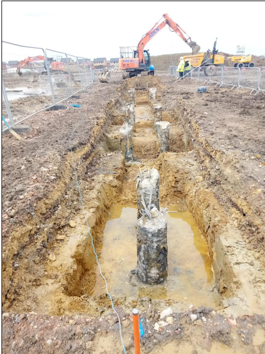
Figure 12. The water table was hit from time to time when the new footings were being excavated, and pumps had to be brought in to remove the water. North facing photo.
