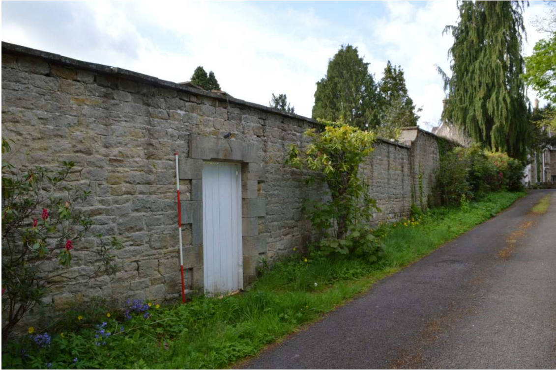
Plate 2: View of northwest garden wall exterior and doorway along-side the driveway to Beauclerc House, facing southwest
