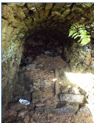
Figure: 33 The entrance to the Kinning Mine Level [GS6]. The tunnel entrance has collapsed further in.
