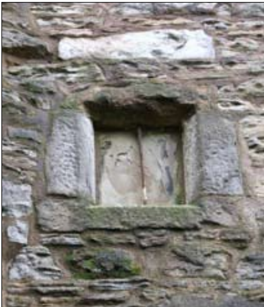
Fig. 28: Small chamfered window with iron bar on the rear of the former library, Front St, Alston, seen from the rear. [DPI35368].
