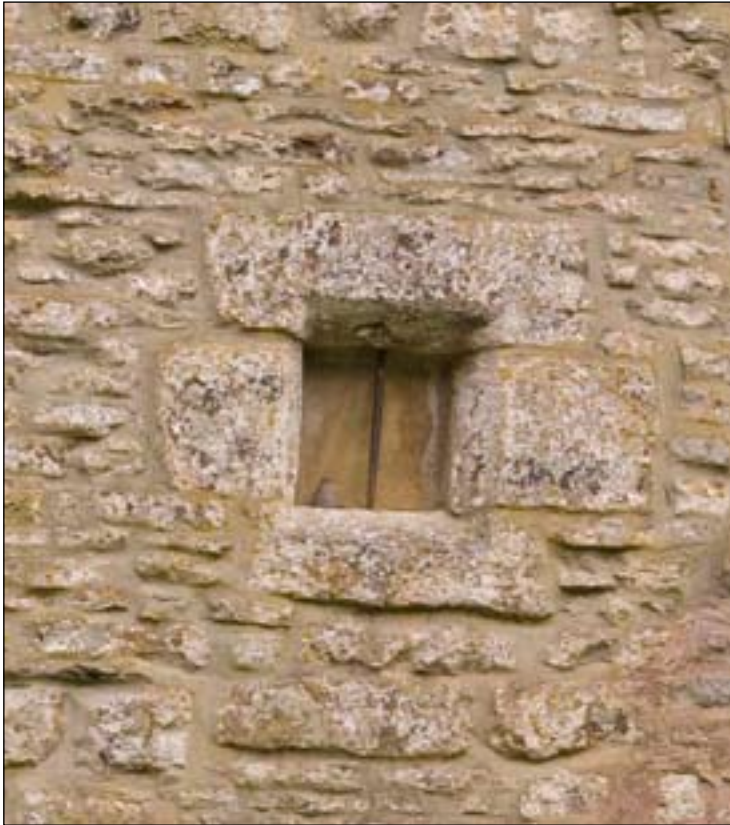
Fig. 9: sandstone rubble walling with ashlar dressings at Nettle Hall, Galligill; probably early 17th century. [DP072082]
