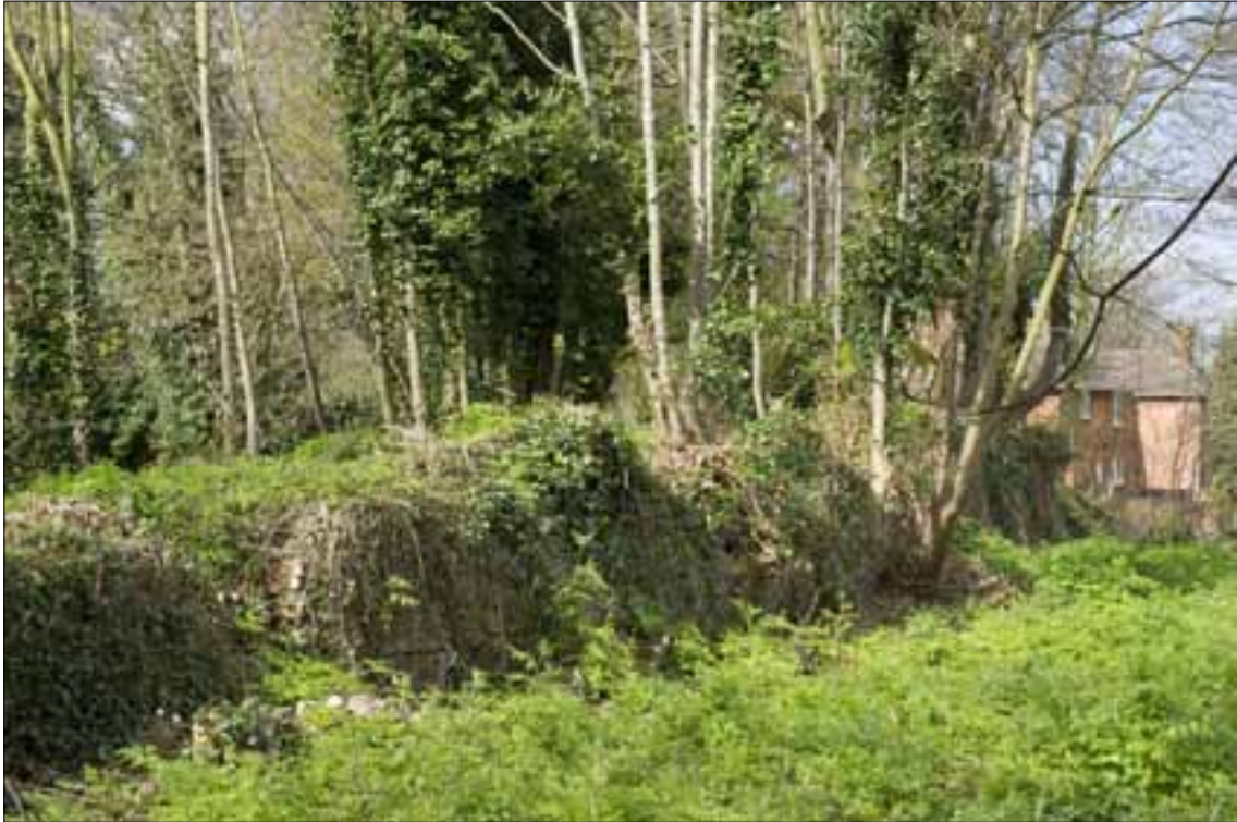
Figure 26 – The parapet revetment along the south flank, from the east (© English Heritage DPI 19301 Steve Cole). The gap visible to the left is damage rather than an embrasure.
