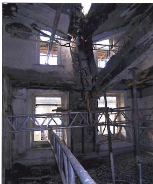
Figure 4. The first floor interior showing the recently collapsed roof internal beams. Pete Smith 5/10/2006
