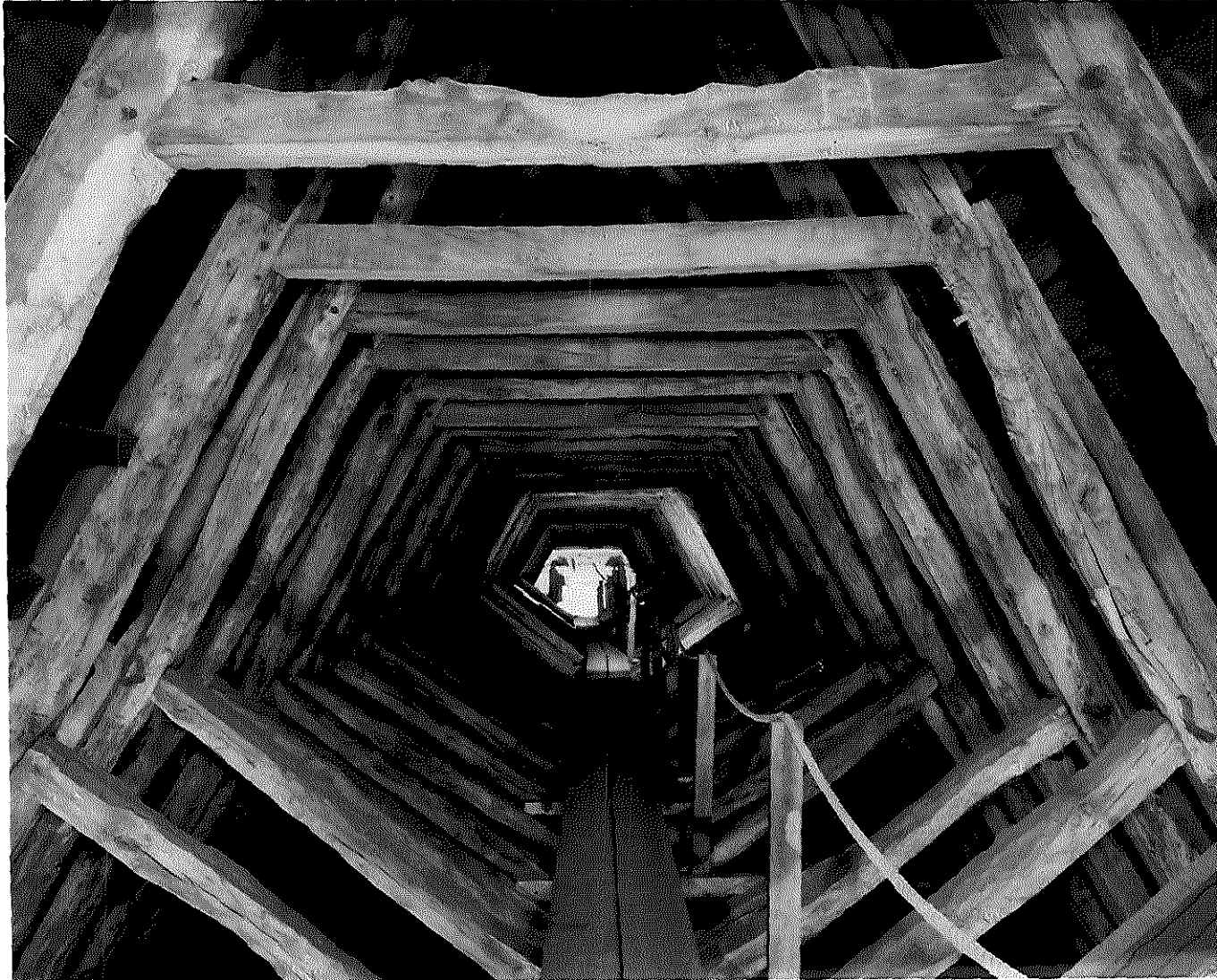
Figure 3a: View of the nave roof looking west to east at walk-way level. (© Crown copyright. NMR. BB87/7303)
