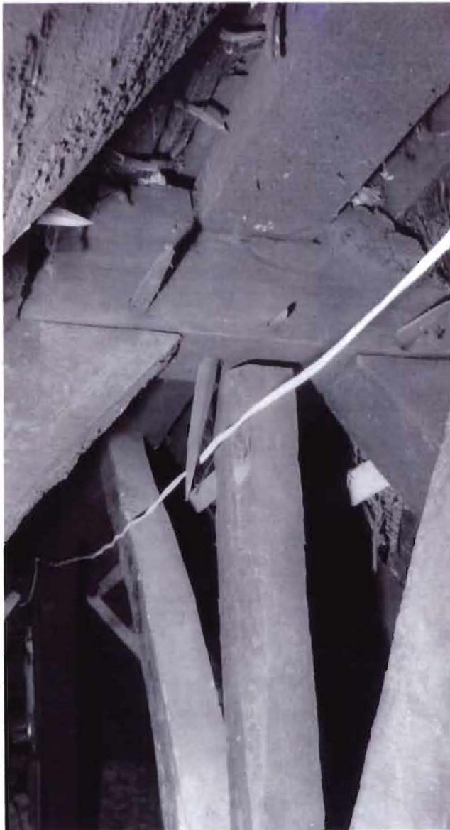
Figure 3c Old Rectory, Cheriton Bishop: truss 3 from the west (photograph J R L Thorp)
