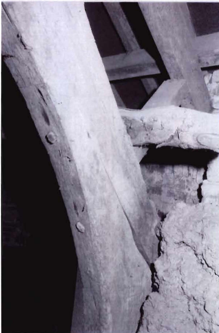
Figure 3m Cleavanger, Nymet Rowland: truss 1 from the west (photograph J R L Thorp)
