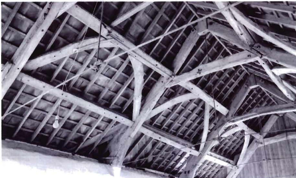
Figure 3t Glebe House barn, Whitestone: trusses 2 to 5 from the north-west (photograph J R L Thorp)
