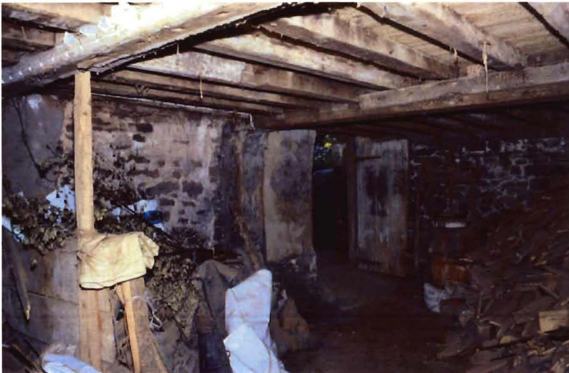
Figure 3p Prowse farmhouse solar cross-wing, Sandford: ground floor looking north-west (photograph J R L Thorp)
