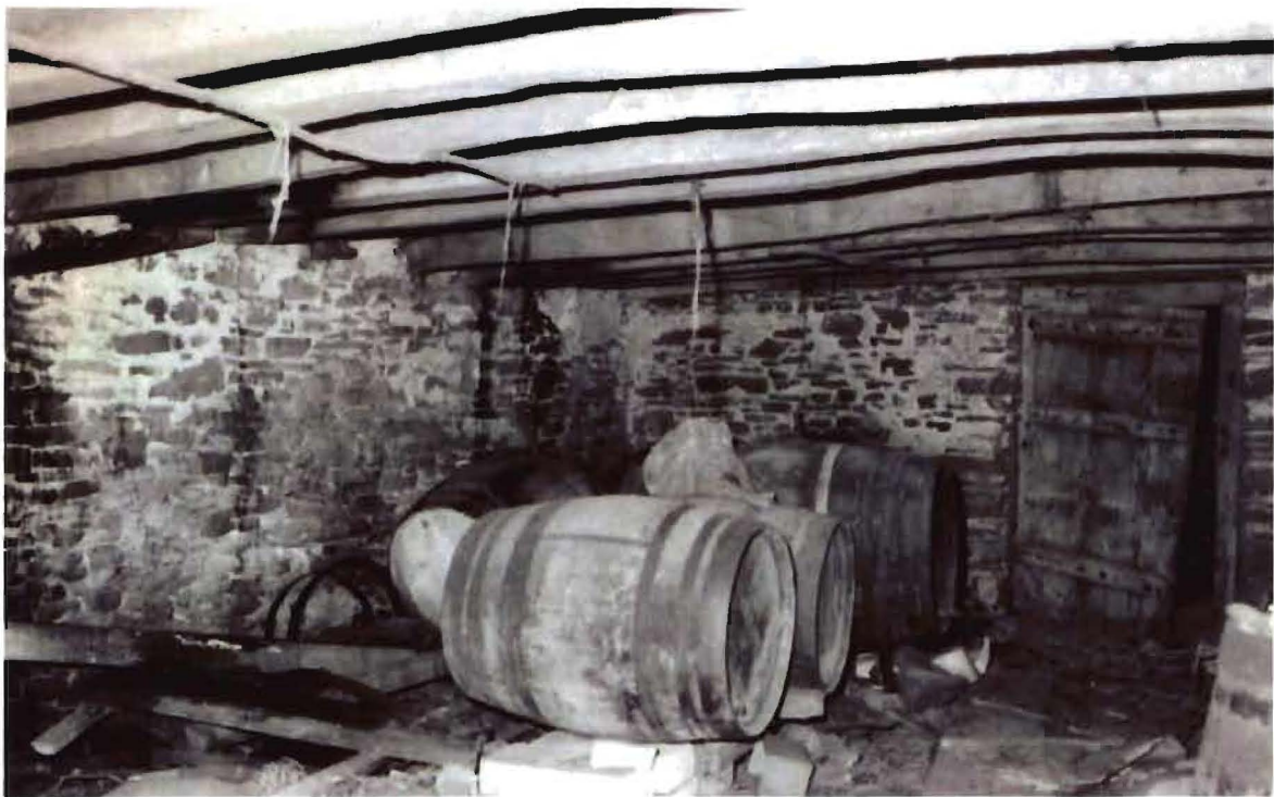
Figure 3h Broomham, King's Nympton: service end or shippon (photograph J R L Thorp)
