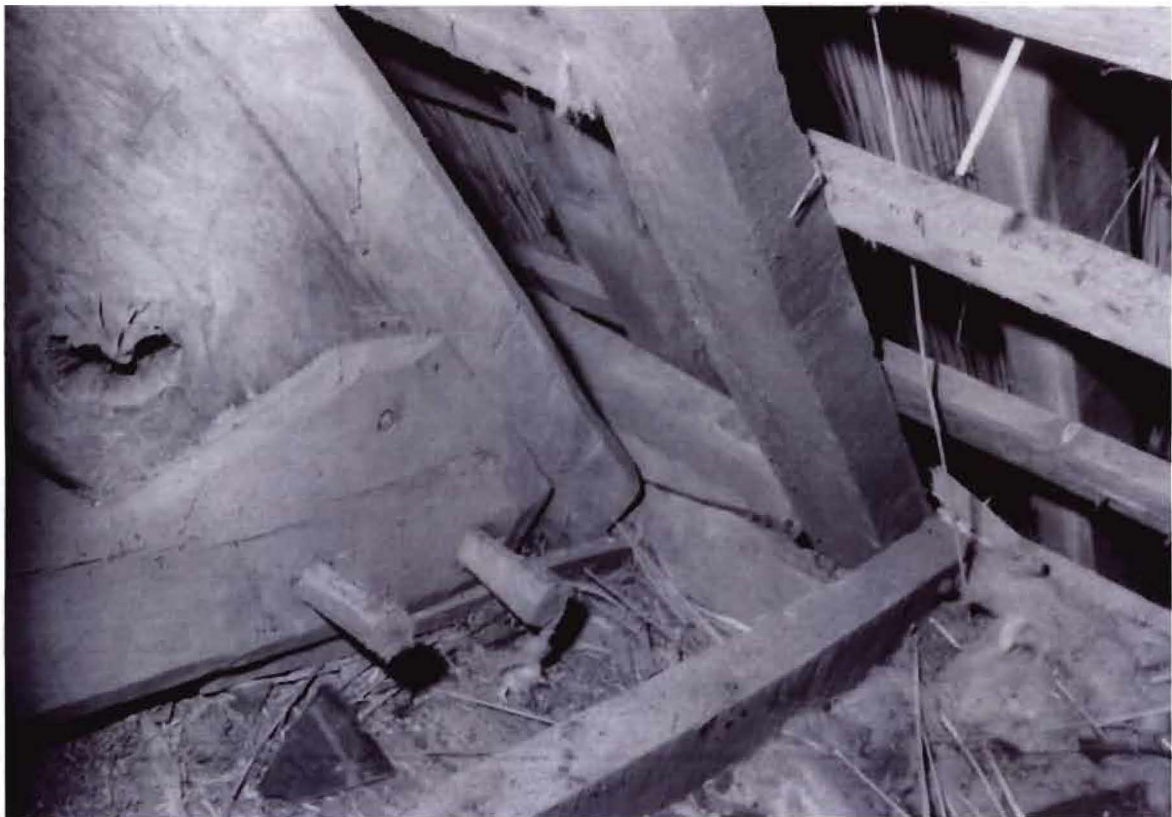
Figure 3g Chaffcombe Manor, Down St Mary: truss 1 from the east (photograph J R L Thorp)
