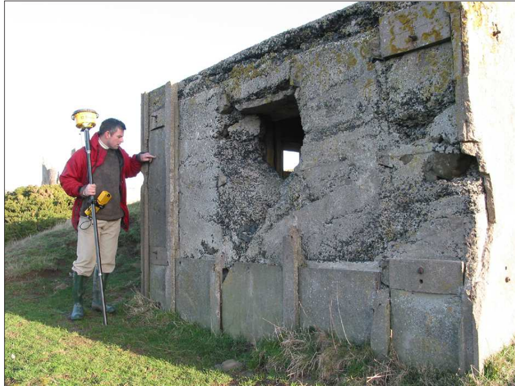
Figure 41. The west side of the pillbox, highlighting bullet impacts resulting from a training attack
