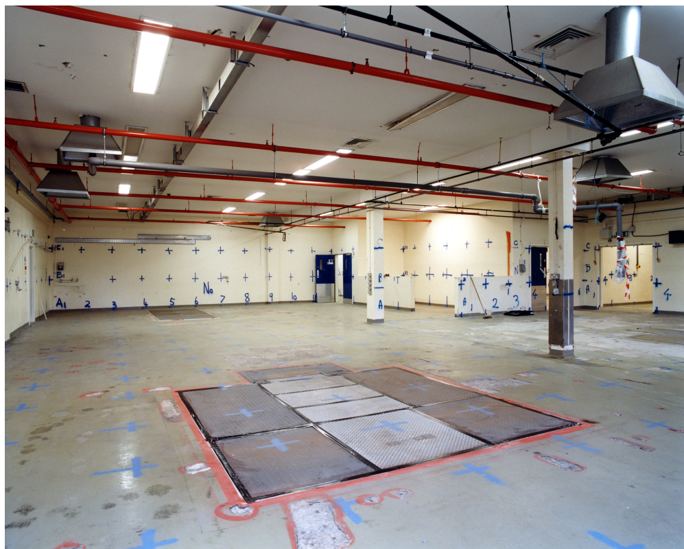
Figure 30 Featherstone, Staffordshire, Royal Ordnance Speciality Metals, one of the depleted uranium machining areas during decontamination operations © English Heritage AA05104
