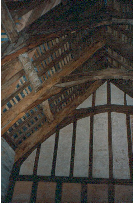
Figure 4 West face of truss T105 in the south range (photograph C Groves)
