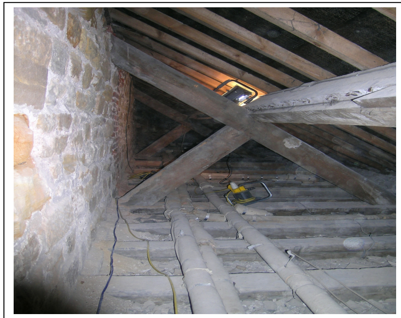
Figure 3a (top): View of a truss from the roof of the main range
