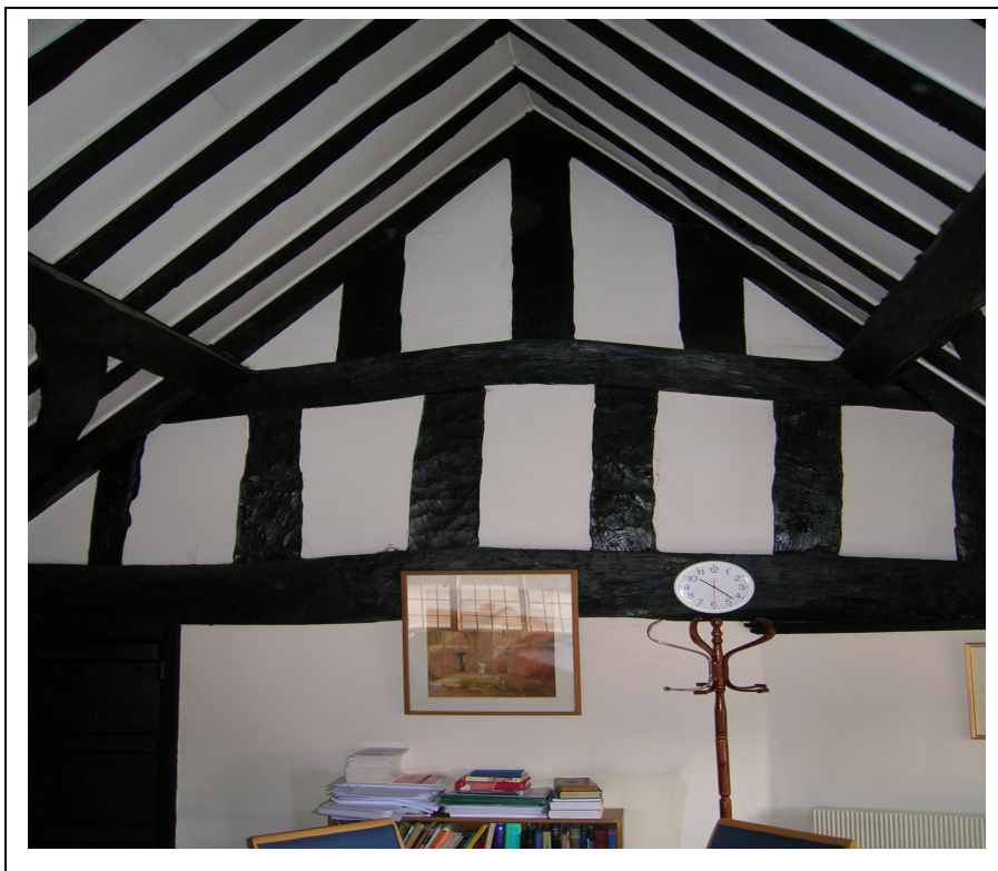
Figure 6a/b: The Pedagogue's House; truss 1 (top), truss 3 (bottom) (viewed from the south looking north)
