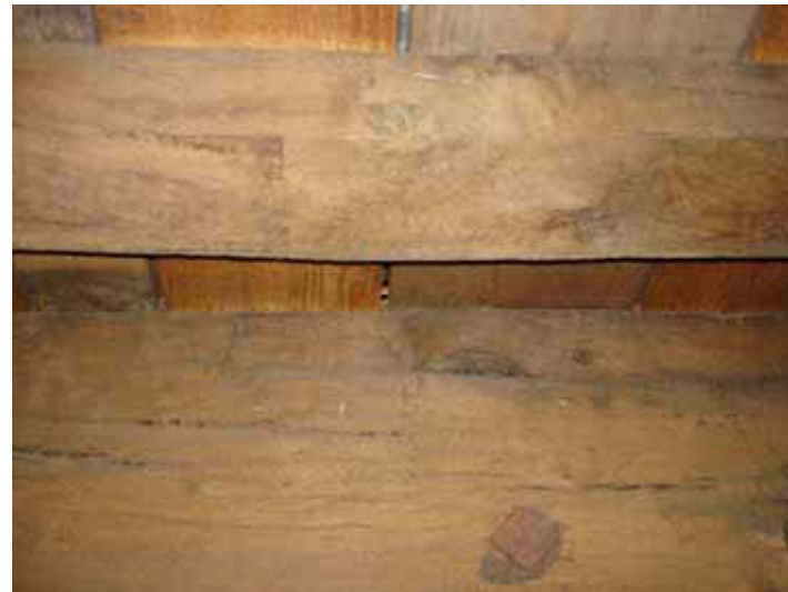
Undersquinted abutment of furring pieces on tiebeam
