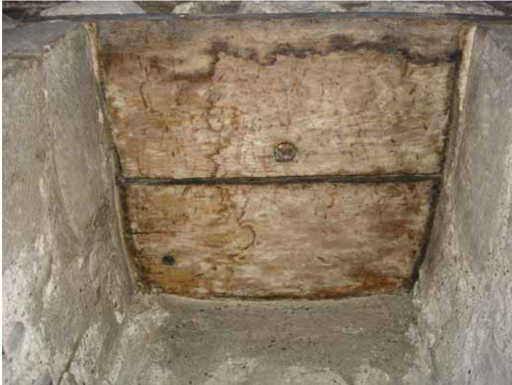
Figure 12: First-floor lintel over cupboard recess in south-east embrasure showing redundant peg hole
