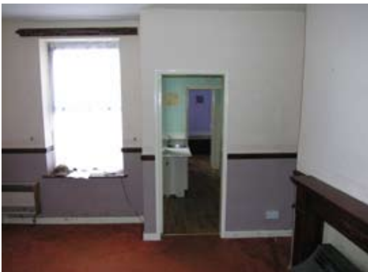
Fig 13: Interior of flat 6A, north-west block, looking from the living room through to the out-rigger. (DPI46638)
