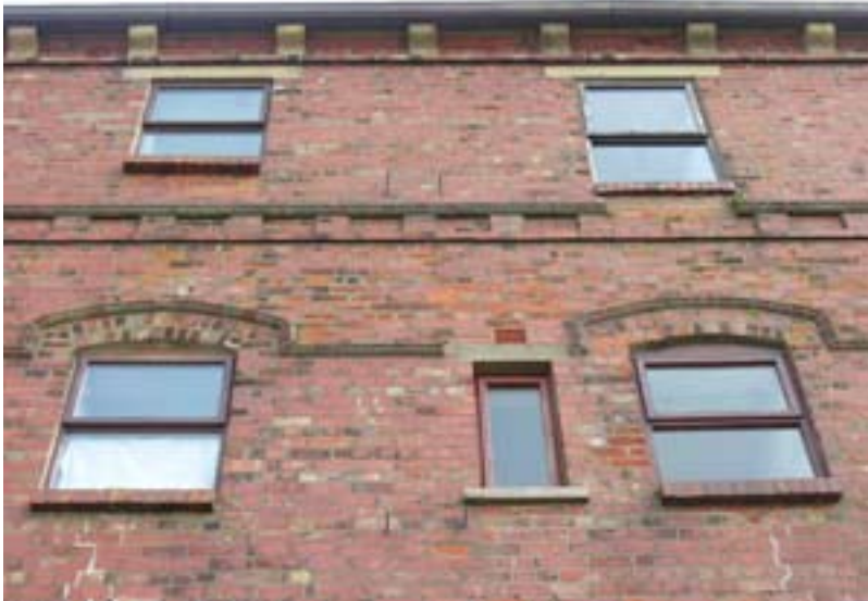
Fig 9: Window details and embellishments on the south-east block, the central window on the lower floor is a late insertion. (DPI46634)
