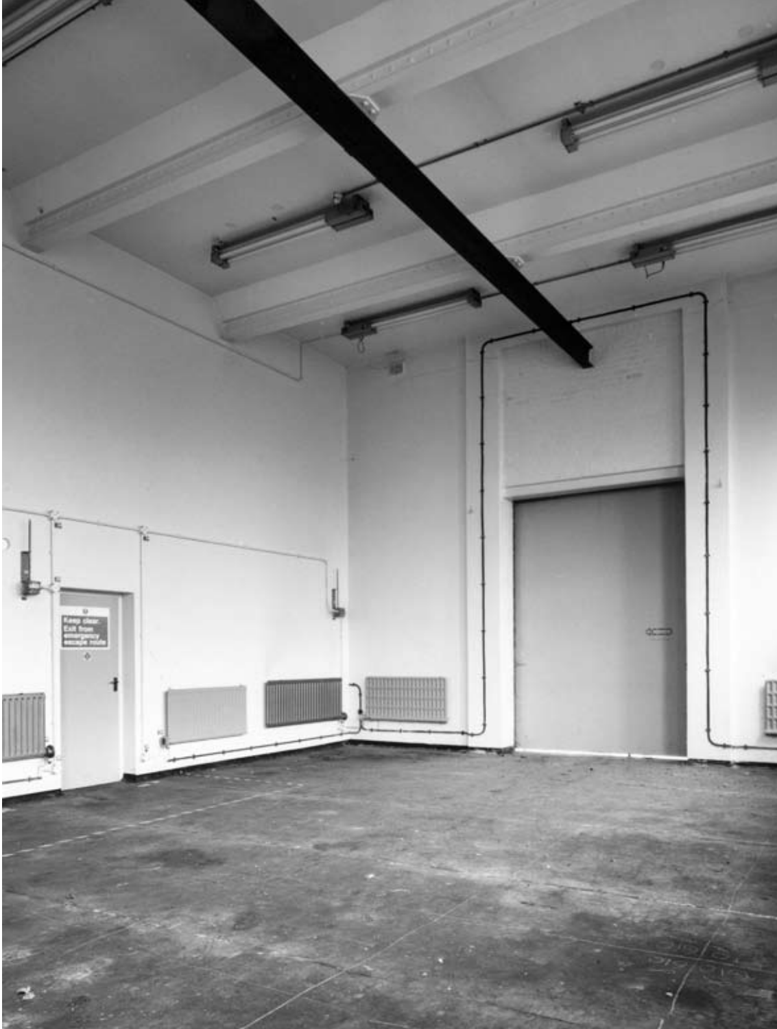
Figure 37: Building X6 was 23, Explosives Preparation Laboratories, interior of Laboratory I showing the main entrance door and over head lifting beam. (c) English Heritage AA99/09785
