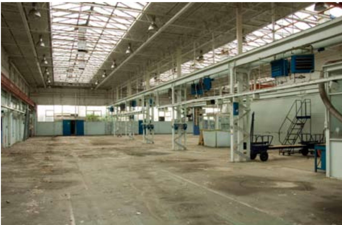
Figure 50: Main Mechanical Workshop E2, northern bay showing its steel framework construction and roof trusses formed from steel sections with tubular steel struts. (c) English Heritage DP035920
