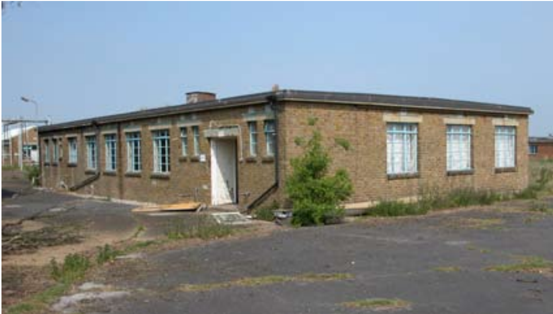
Figure 46: Canteen A7, was 24, is typical of buildings of this date with brick walls, a flat concrete roof, metal Crittall windows with concrete lintels and sloping brick sills. (c) English Heritage
