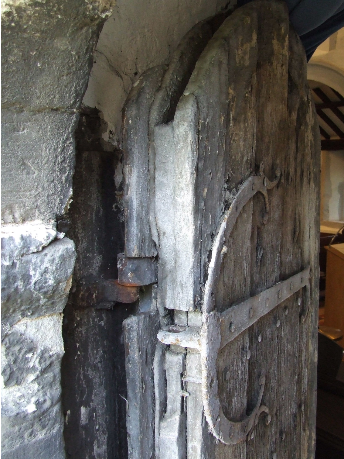
Figure 4. View of the door showing the front boards, the ironwork, the original pintle, the very thin rear boards, and the thicker rear cladding and present pintle
