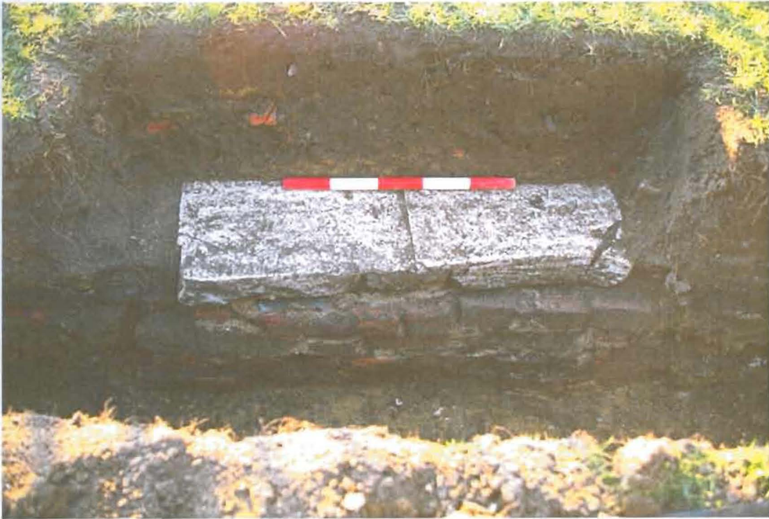
Figure 12. Photograph showing one of the three brick manholes/inspection shafts capped with Portland limestone slabs (context 127 - see figure 5)
