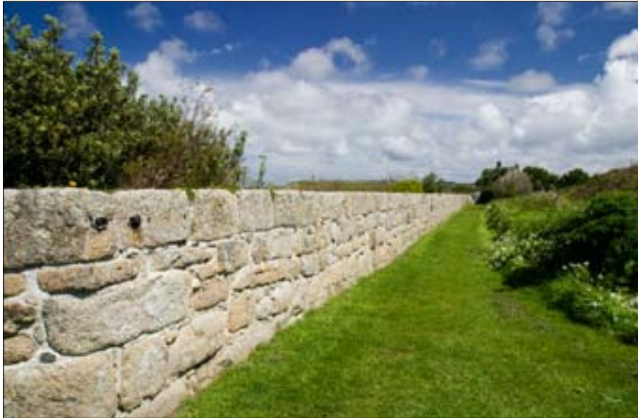
Figure 26. Wall between King Charles' Battery and Newman's on north side of the Garrison. [DP022513]
