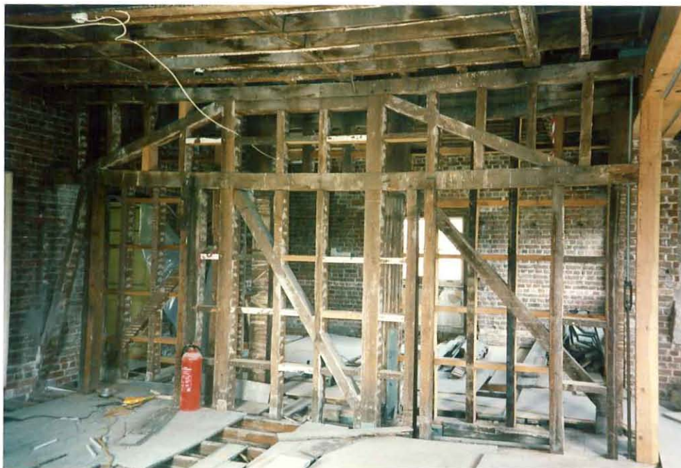
Figure 10: Photograph of south face of partition E, with partition F behind on the bedroom level (C Groves)
