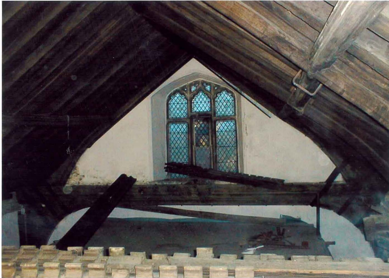
Figure 2: View of the nave roof showing moulded purlins and principal rafter and embattled tie beam (photo A F Knight Builders of Debenham)
