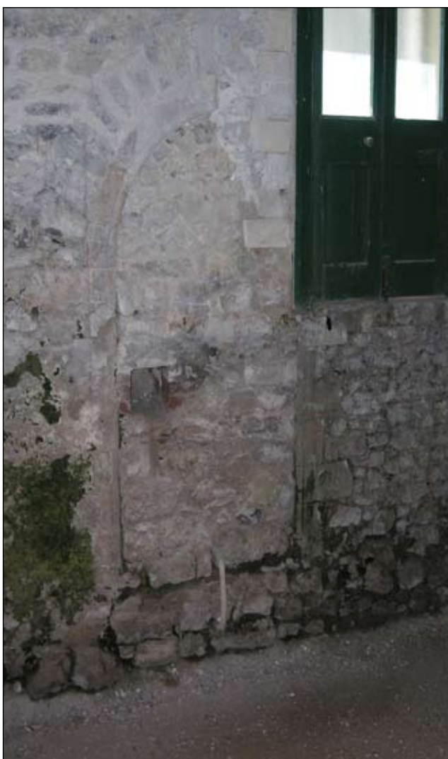
Figure 5. Blocked doorway at upper end of hall
