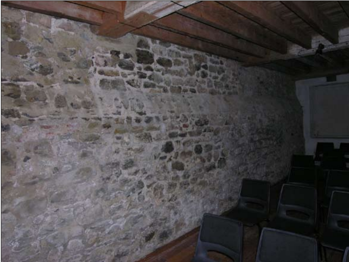
Figure 9. Battered wall on inside of AV room (former external face of kitchen wall)
