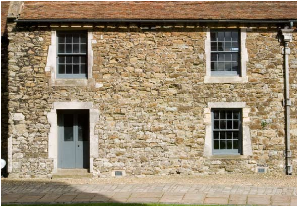
Figure 16. Joint between regular 18th-century fabric and medieval rubble, to left of right-hand sashes
