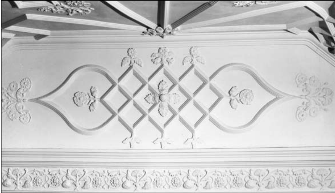
Figure 25. Detail of plasterwork on north wall of first-floor room of north wing (BB96/3912).
