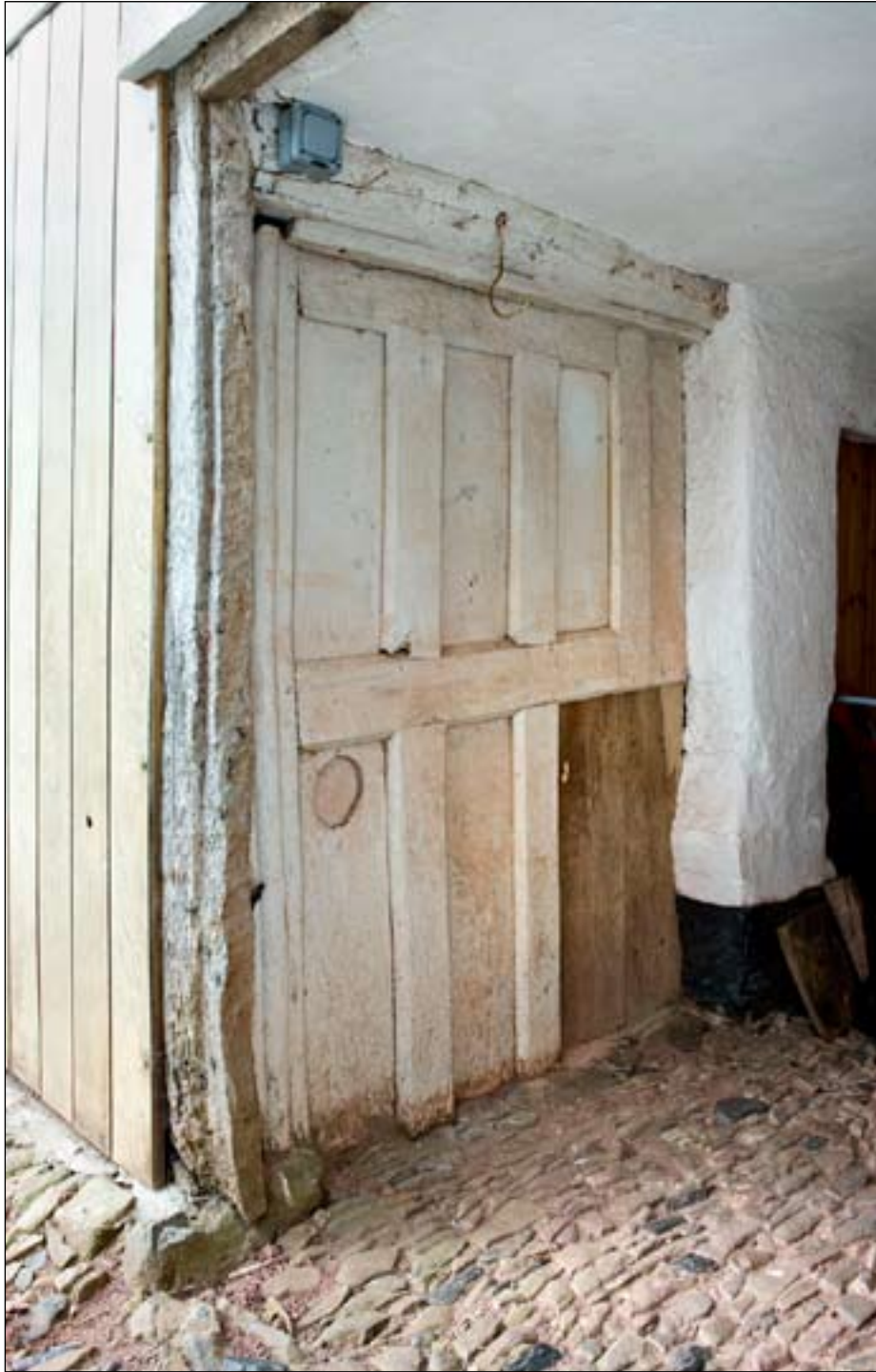
Figure 15. Panelled screen, probably part of the former screens passage, re-used in the linhay (DP113800).
