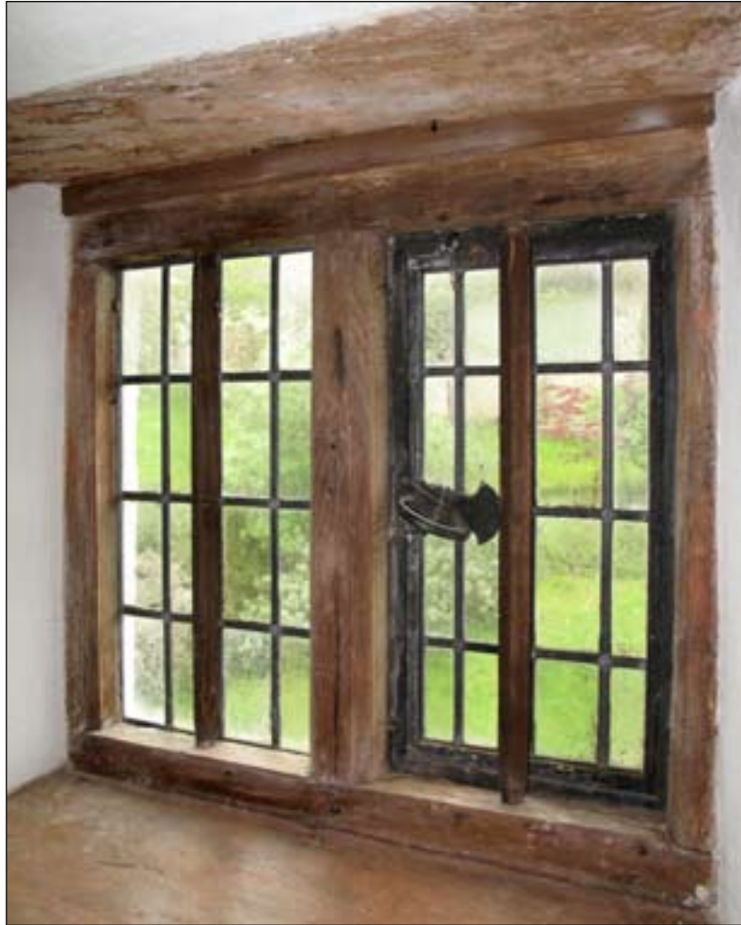
Figure 12. Two-light window in eastern wall of bay D-E, with chamfered mullions and jambs, probably dating to the late 16th or early 17th century (DPI13788).
