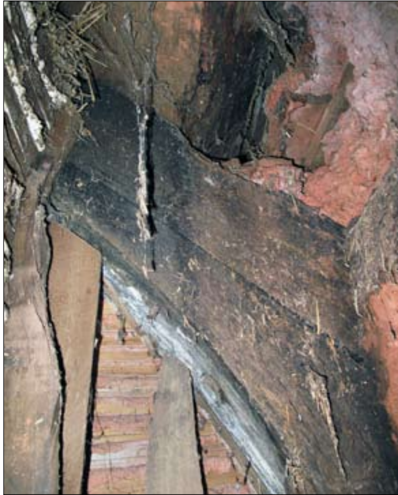
Figure 11. Detail of northern foot of cruck C-CI showing jointed-cruck construction and face-pegging (DP113780).
