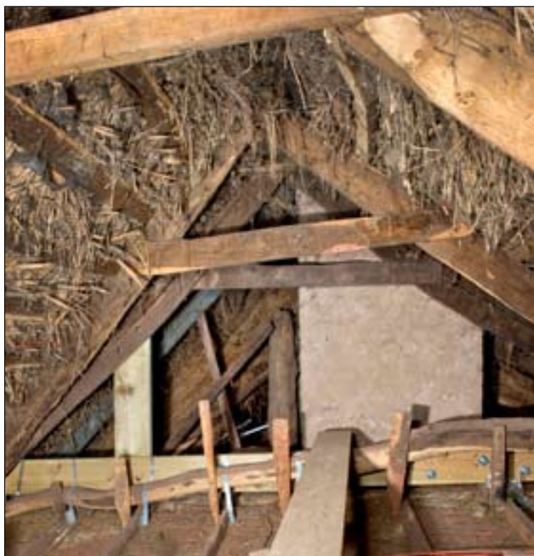
Figure 4. Roof space looking west to former position of cruck truss B-B1, showing inserted chimney stack (DPI13792).
