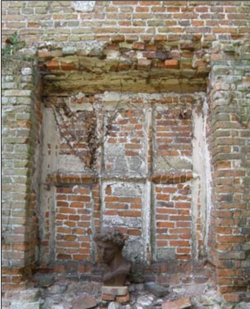
Fig. 36. One of the blocked windows in the surviving brick front wall to the south range of Lord Darcy's former house.
