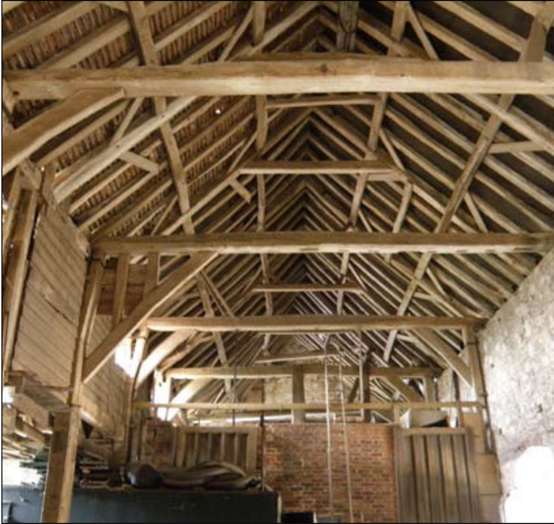
Fig. 6. The interior of the mid-16th century timber-framed Tithe Barn looking west. © Pete Smith P5132878.JPG
