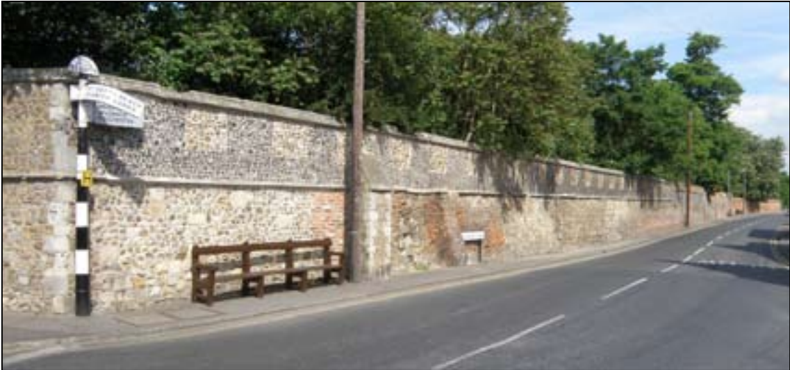
Fig. 37. The much repaired and restored Boundary Wall running along the east side of the park and the west side of Colchester Road. © Pete Smith P5132804A
