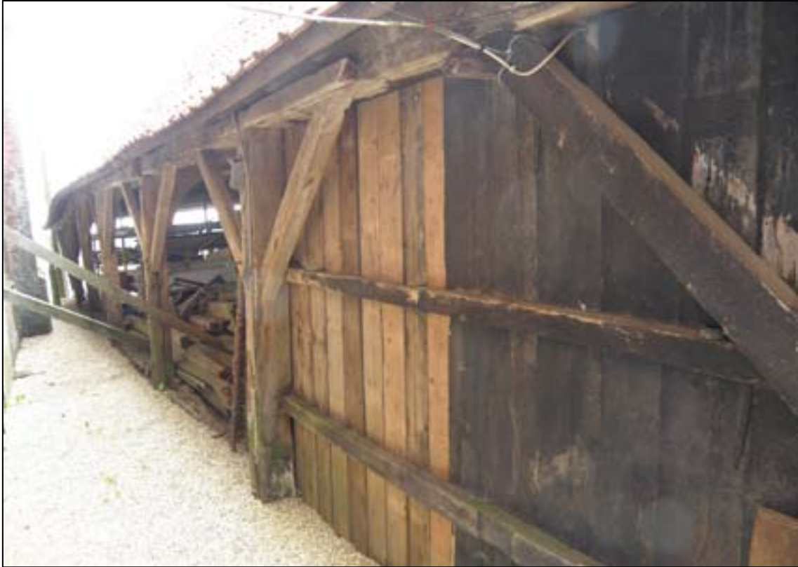
Fig. 8. The late 18th century timber-framed Cartshed, probably moved to its present site in the late 19th century. © Pete Smith P5132882.JPG
