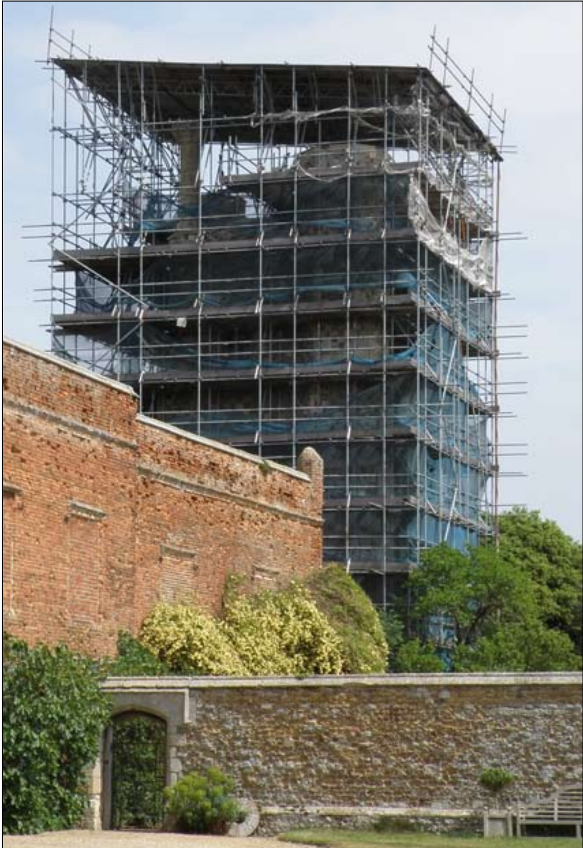
Fig. 29. The Abbot's Tower at present clad in scaffolding and undergoing restoration. © Pete Smith P5132915A.JPG
