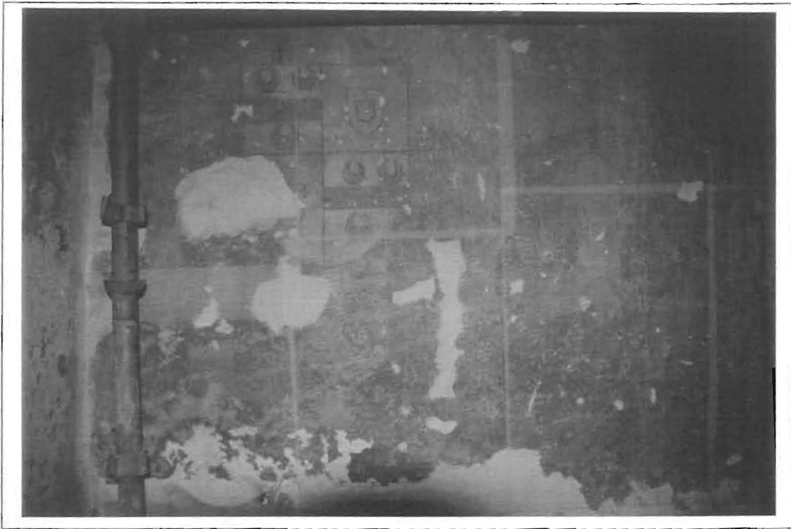
South wall, east side, area of fictive tapestry and heraldry, before removal of tissue facing and Polyfilla repairs, May 1996
