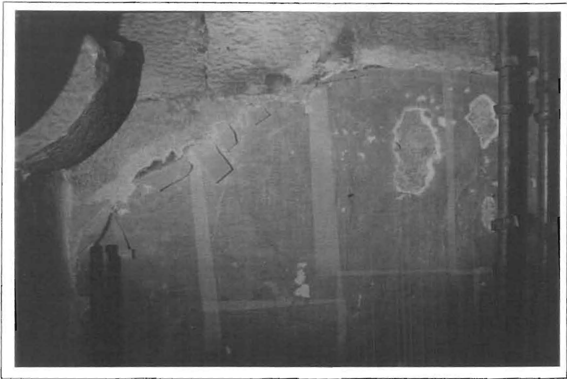
South wall, east side, naval scene, before removal of tissue facing and Polyfilla repairs, May 1996
