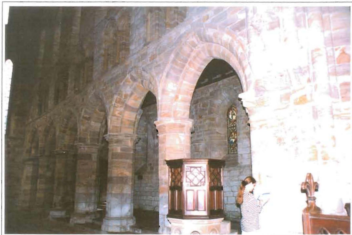
Nave, north side, looking northwest: fragment of painting located on NW pier of crossing, seen on right side of the photograph
