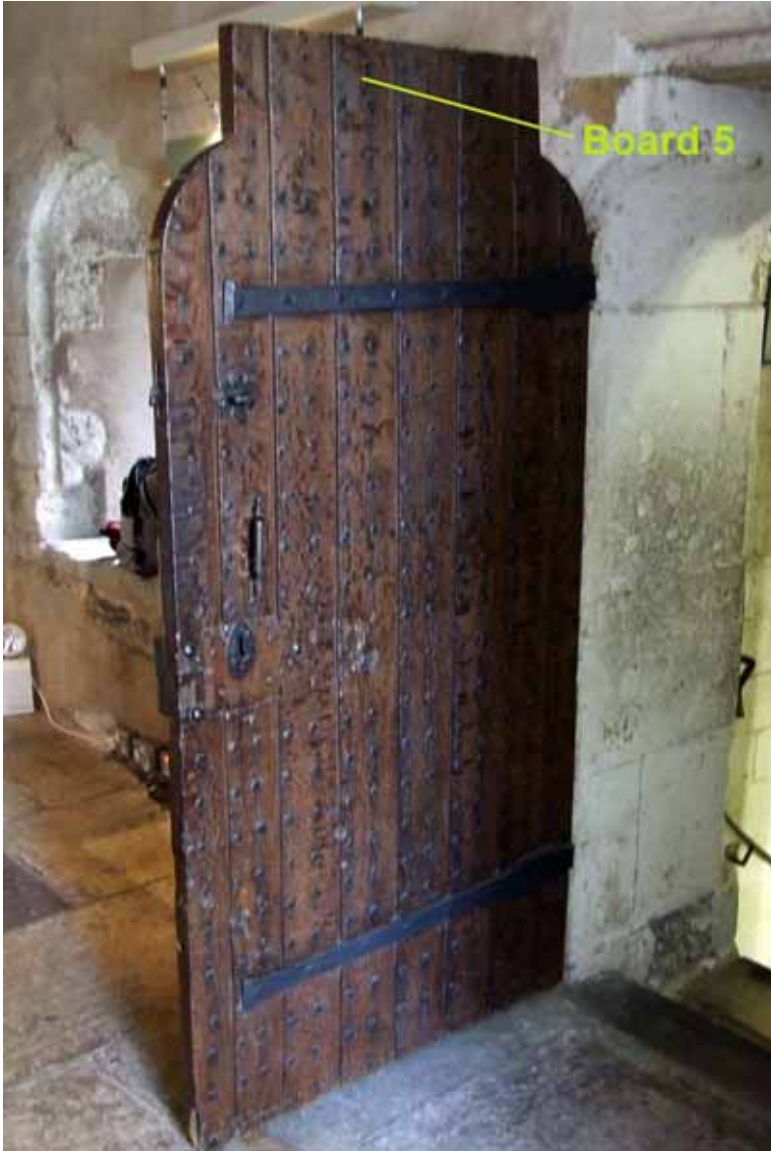
Figure 4: The door to the second floor chamber, indicating the position of the dated board
