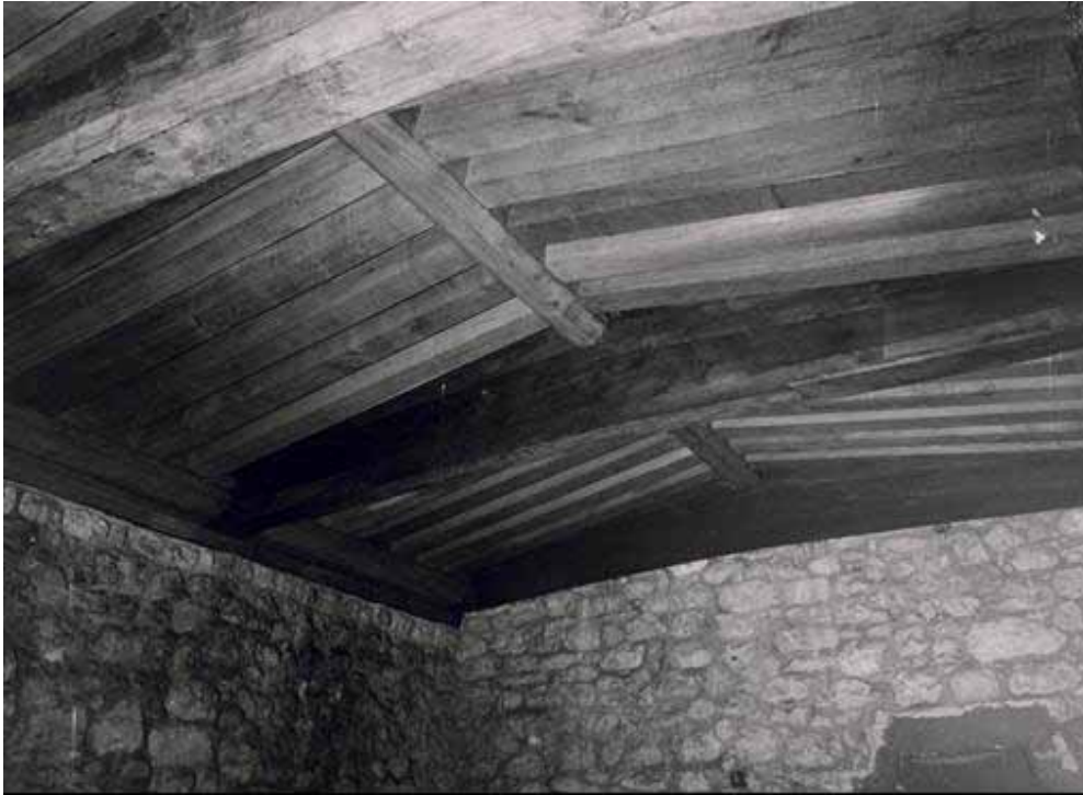
Figure 2: The roof of the main upper chamber (photograph from the National Monuments Record)
