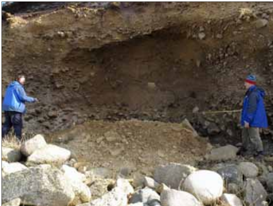
PI 35: Allan Brodie and the author measuring erosion undercutting the cliffs on the Garrison. (EH NMR DP116017: 9 March 2010)
