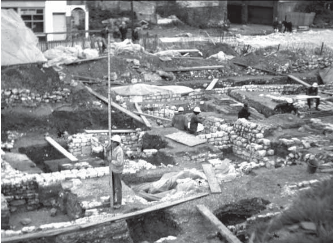
Figure 14 – At York Street, Dover, excavations before bypass construction by Kent Archaeological Rescue Unit led by Brian Philp, revealed important Roman remains including the Painted House (open to the public in New Street) and the base for the Classis Britannica , now buried under the road and the Discovery Centre (courtesy of Dover Museum & Bronze Age Boat Gallery, www.dover.gov.uk/museum ).
