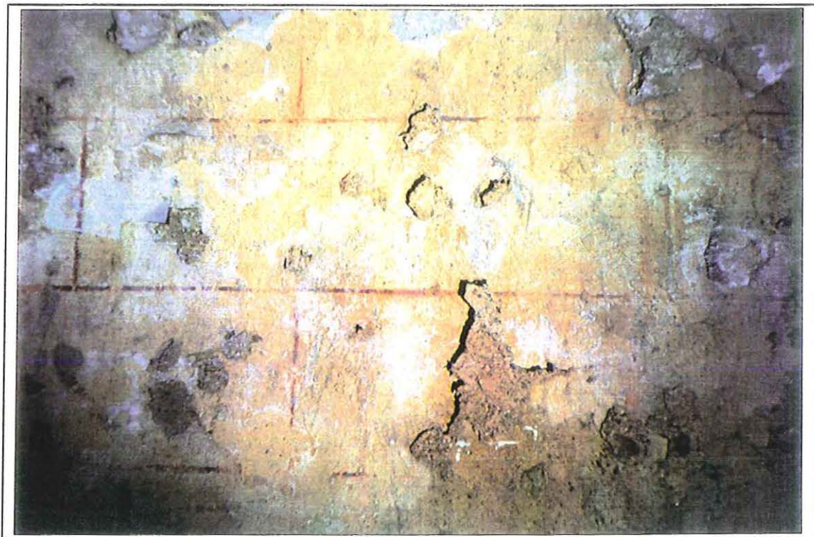
Dorter, north wall, detail of single red-line masonry pattern, before conservation in 1993
