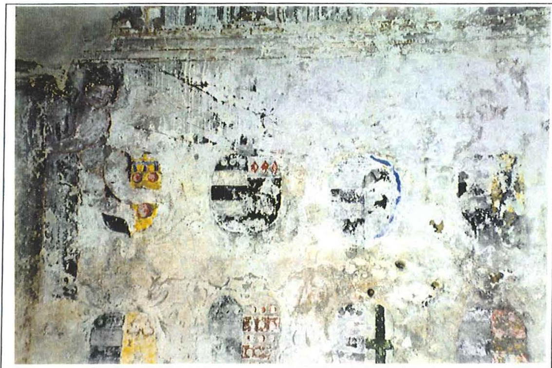
St Anne's Chapel, north wall, detail of 17C decoration with later (19C) additions
