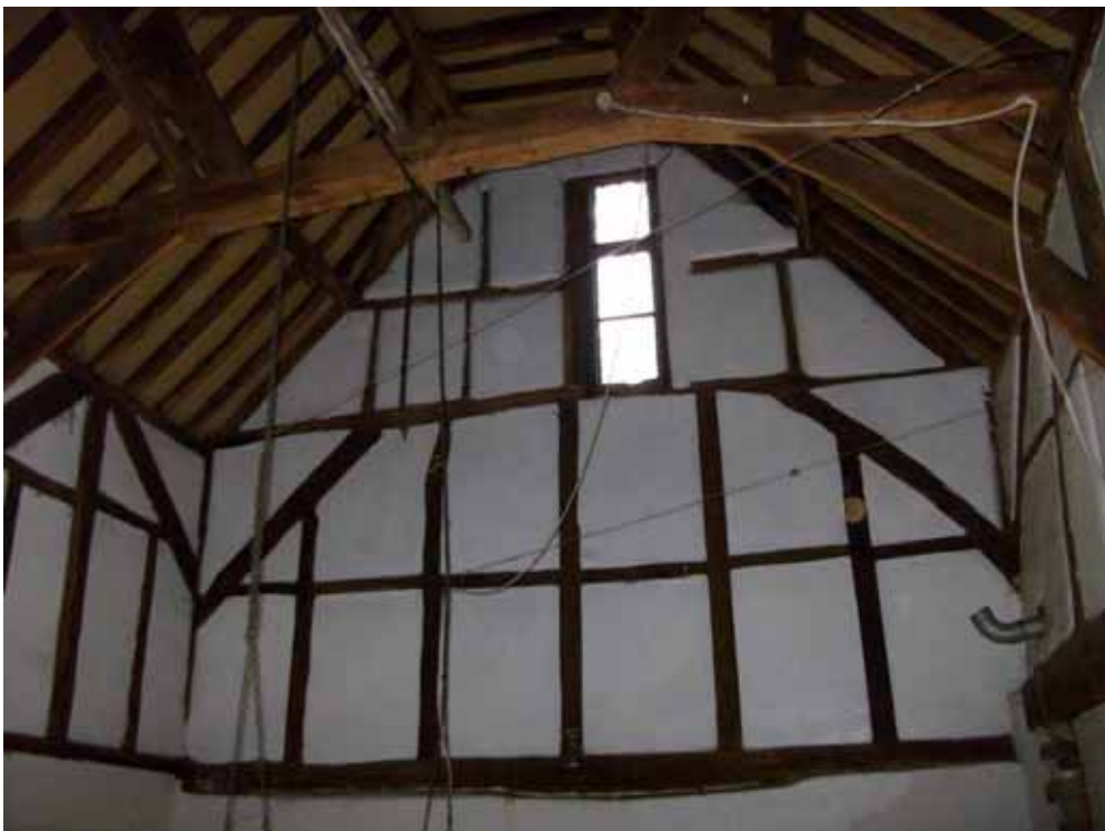
Figure 4a/b: General internal views of the Old Coach House, looking site north to south (top), and south to north (bottom)
