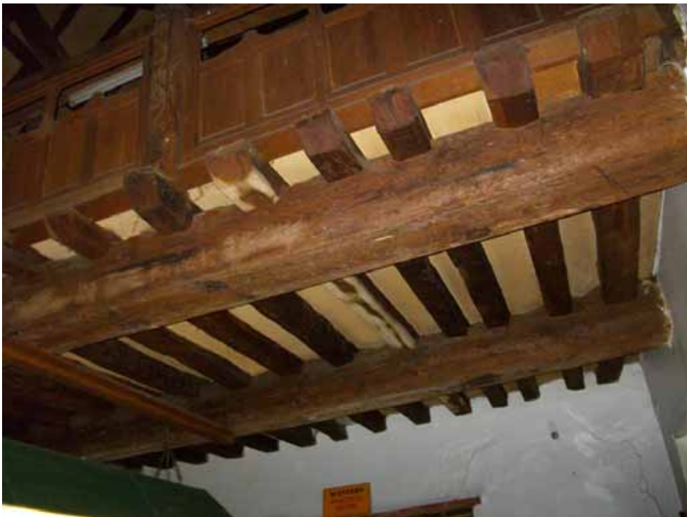
Figure 4c/d: Views of the roof (top) and the beams of the gallery (bottom)
