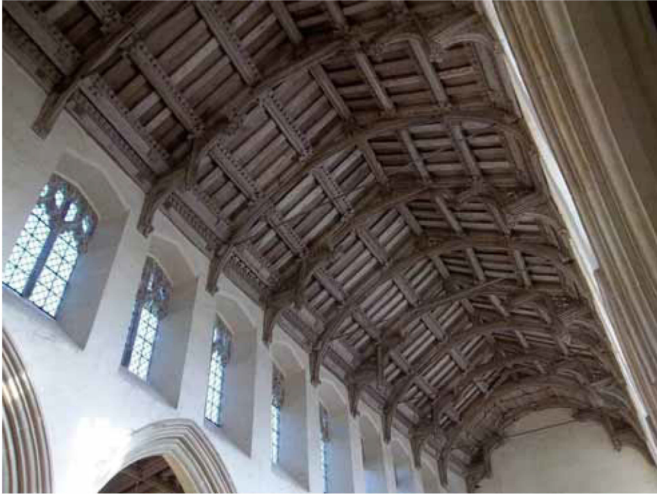
Figure 3a: View of the nave roof showing the alternating double hammer beam and arch-braced trusses
