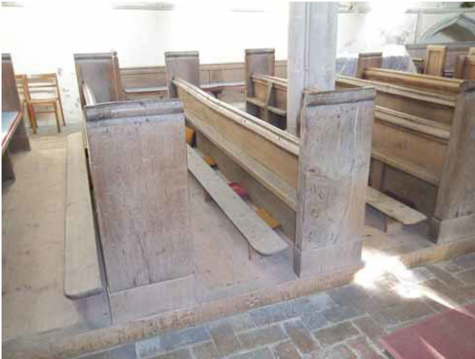
Figure 4b: Detail of the bench ends of the early pews
