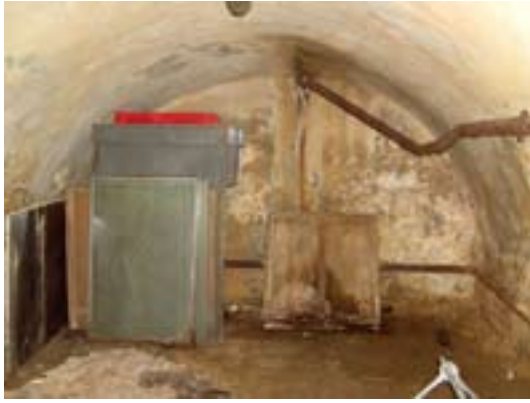
Figure 32 One of the coal cellars of 1–2 Montague Place. Copyright English Heritage (DP070369)
