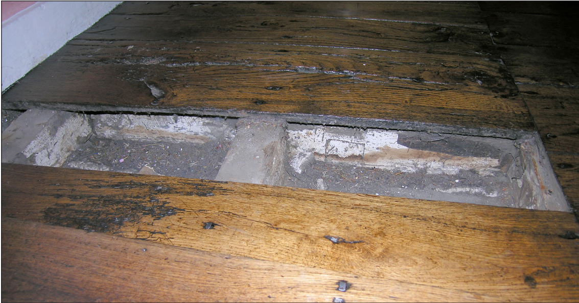
Fig 34: The joisted houseplace ceiling, exposed by lifting floor boards in the room above, showing limewashed timbers and traces of paper [AM]
