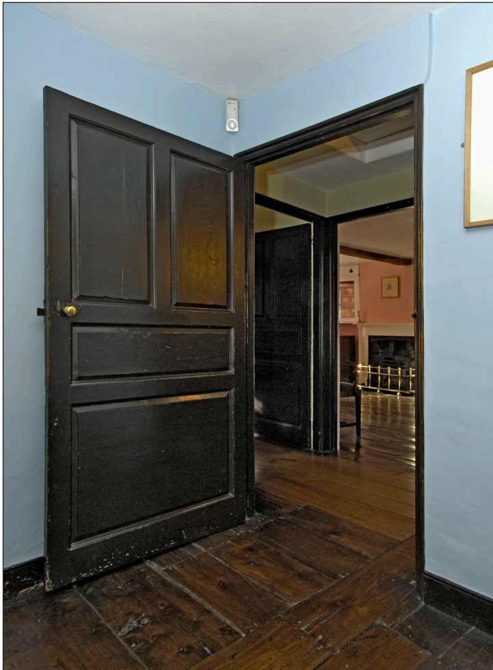
Fig 14: The early to mid-18th-century door to the rear bedroom, looking across the landing to the north-west bedroom (Wordsworth's Sitting Room) [dp056093]
