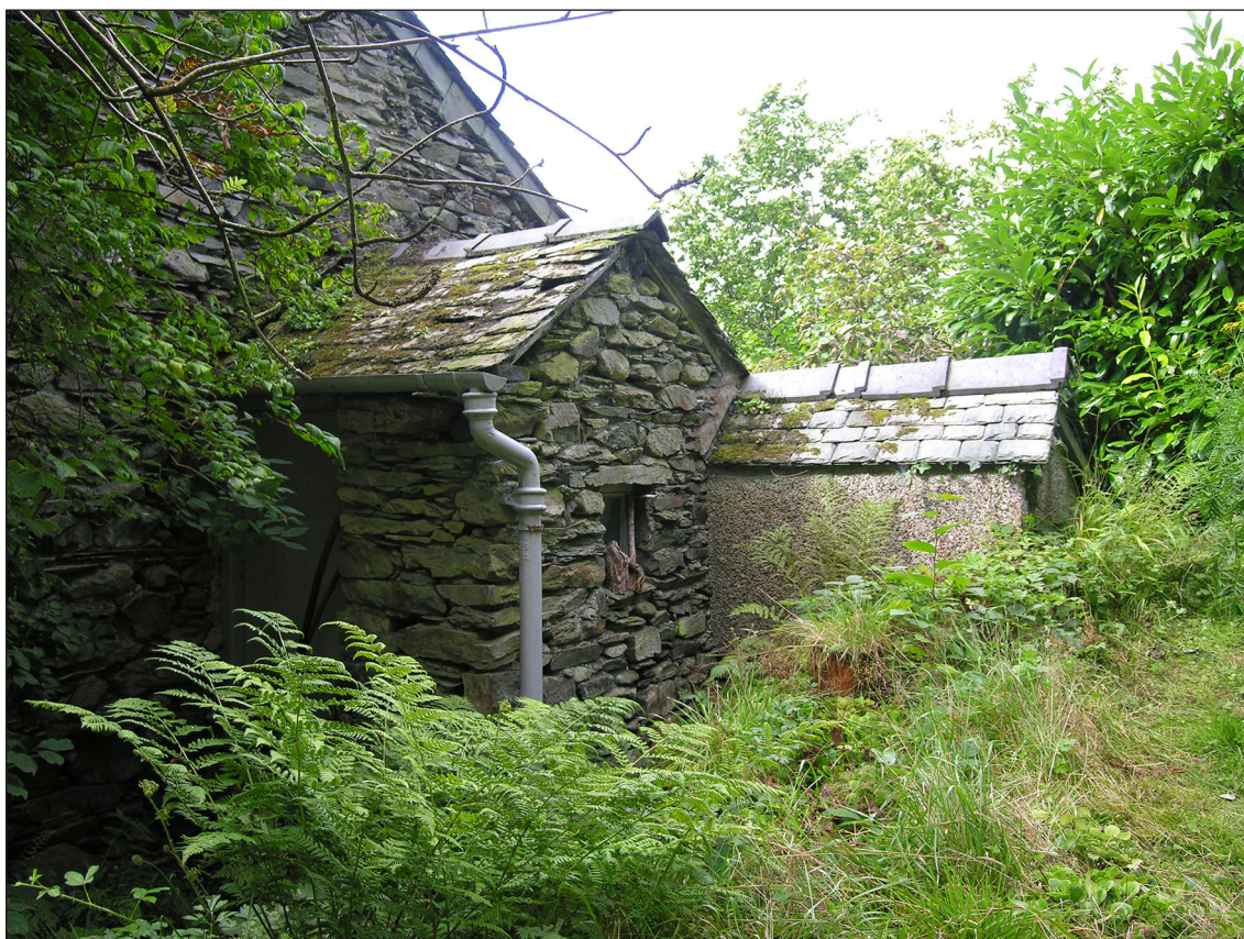
Fig 52: The Necessary House (with the small window) from the east; the entrance is to the left. The upper portion of the Museum Wing is further left and the lower roughcast structure to the right is the Boiler Room of 1928 [AM]
