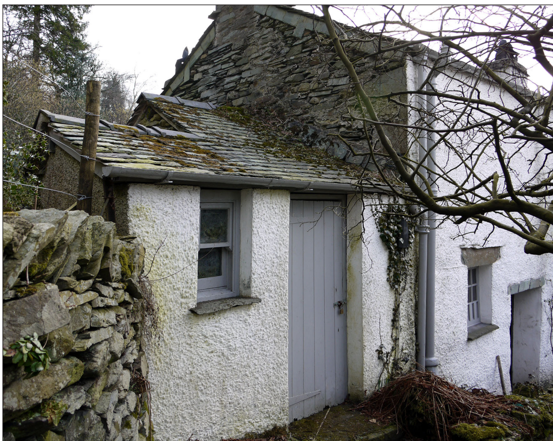
Fig 53: The Boiler House of 1928. Pointing to the chimney and gable of the Museum Wing beyond date from the insertion of the boiler flue [AM]
