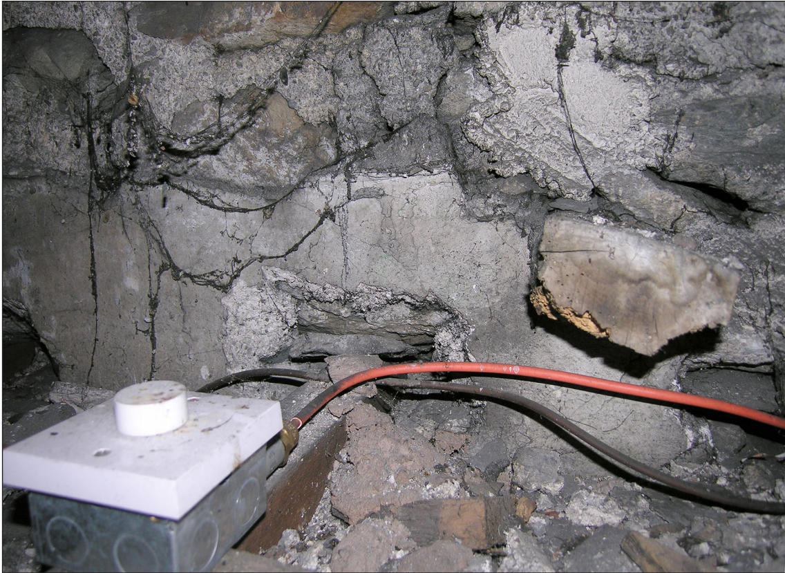
Fig 49: The surviving end of a purlin is associated with a plaster wall surface the upper edge of which rises from the right and runs level to the left of the purlin [AM]
