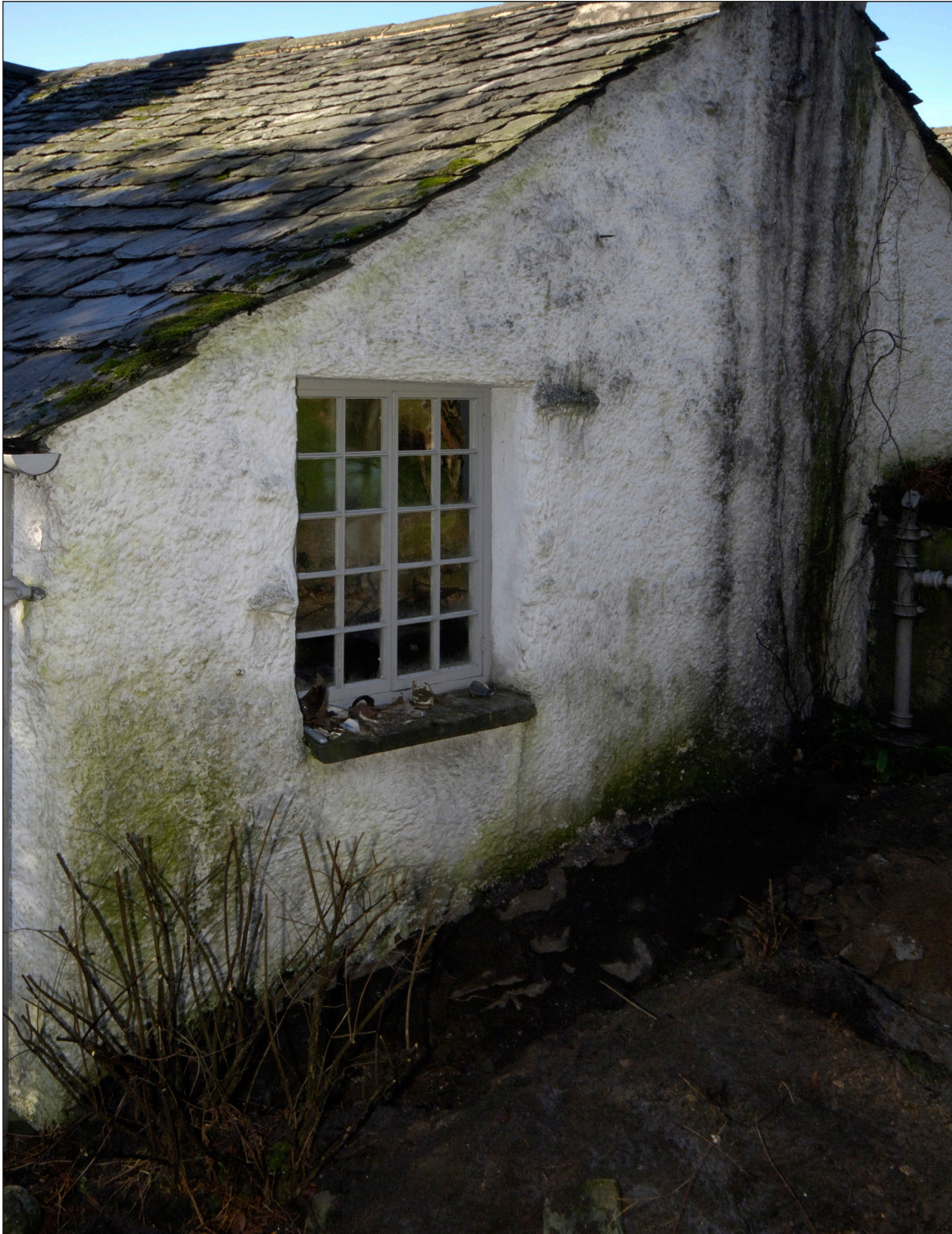
Fig 29: The gable of the rear range, showing the window of the rear bedroom and what may be the remains of a drip course to the right [dp056066]
