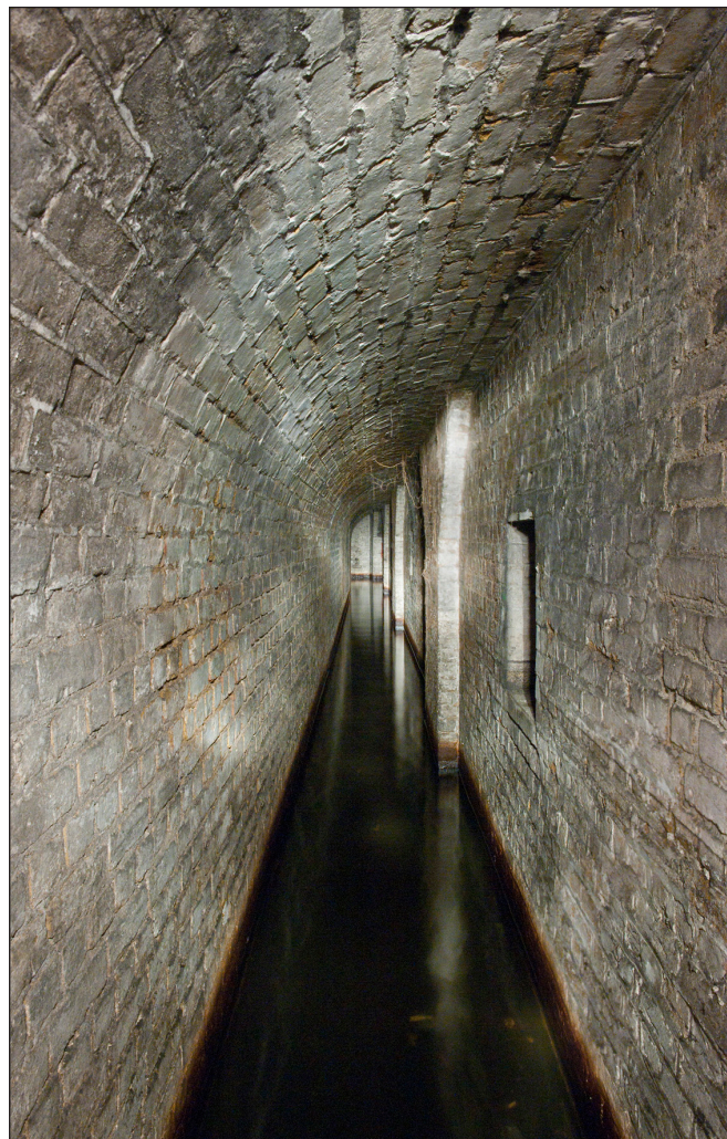
Figure 11: The main lighting passage looking south-west showing the restricted height of the passage and its slightly irregular vault. An opening for the light box in the end wall of the ammunition store can be seen in the wall on the right of the photograph. (DP097416)
