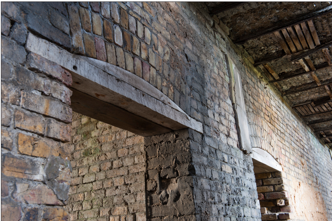
Figure 32: Reinforced door heads and patched cracks in the north wall of the officers' quarters may be evidence of subsidence of the south range. (DP 097474)
