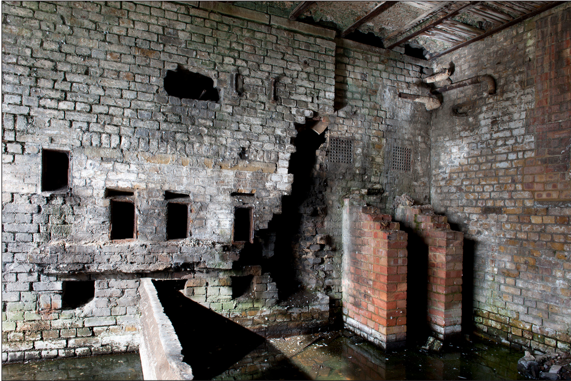
Figure 27: The north wall of the Cook House. The position of the ovens is marked by the iron-framed rectangular openings. Evidence of later reuse can also be seen in the form of the low concrete wall and red-brick boiler footings. (DP097464)
