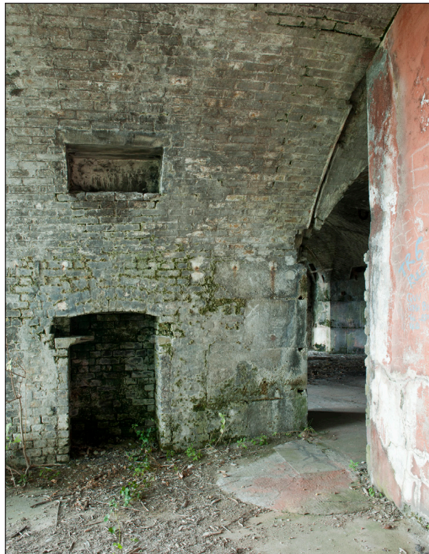
Figure 21: Detail in Casemate 5 of what is thought to be the original fireplace and air vent for the living casemates. The edge of a concrete traverse, painted orange brown, can be seen on the right of the picture. (DP 097601)
