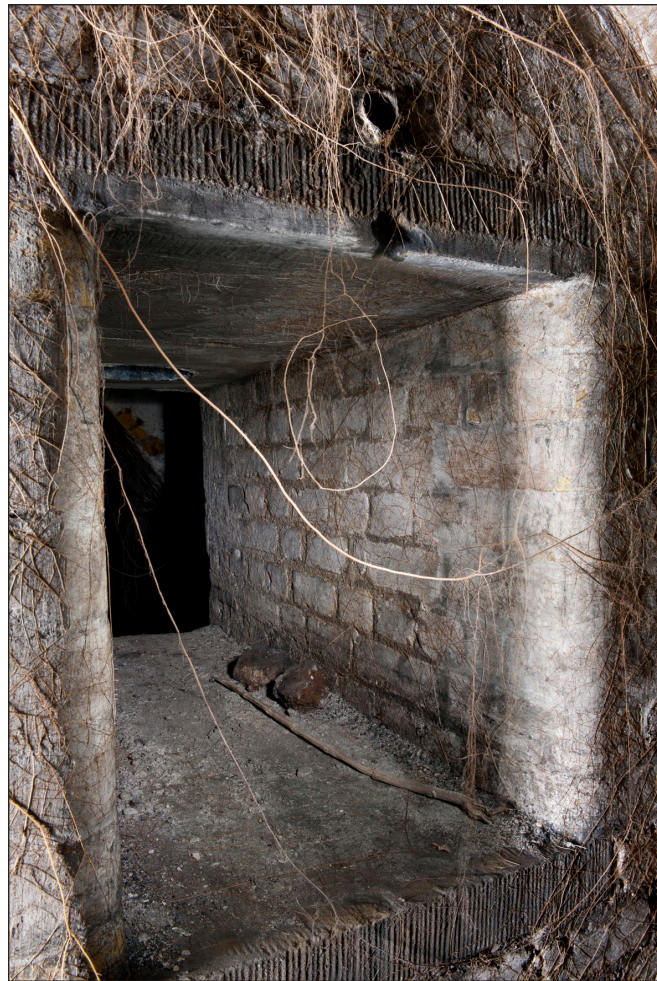
Figure 12: Close up view of a light box from the lighting passage side. The vent pipe positioned just above the masonry lintel provided the oxygen source for the lamp flame. (DP097416)
