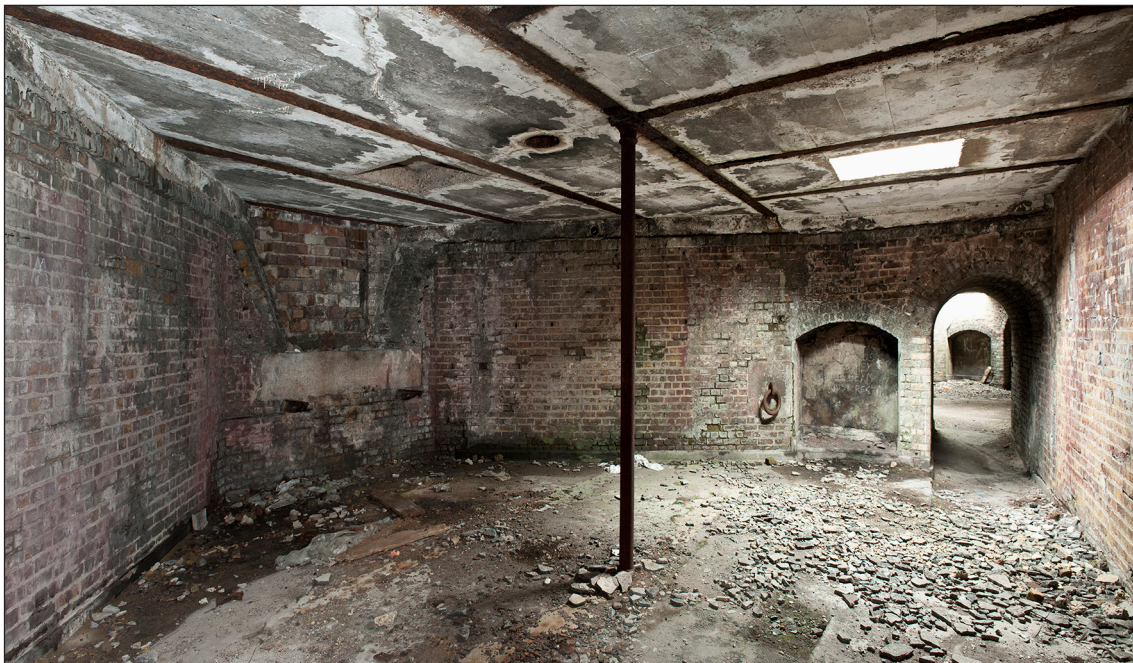
Figure 22: The southern former open gun emplacement looking north towards the second open emplacement. The blocked brick gun embrasure can be seen to the left of the image whilst the ring and set back associated with traversing the gun can be seen to the right adjacent to the passage which connects this emplacement to the one to the north. (DP097650)
