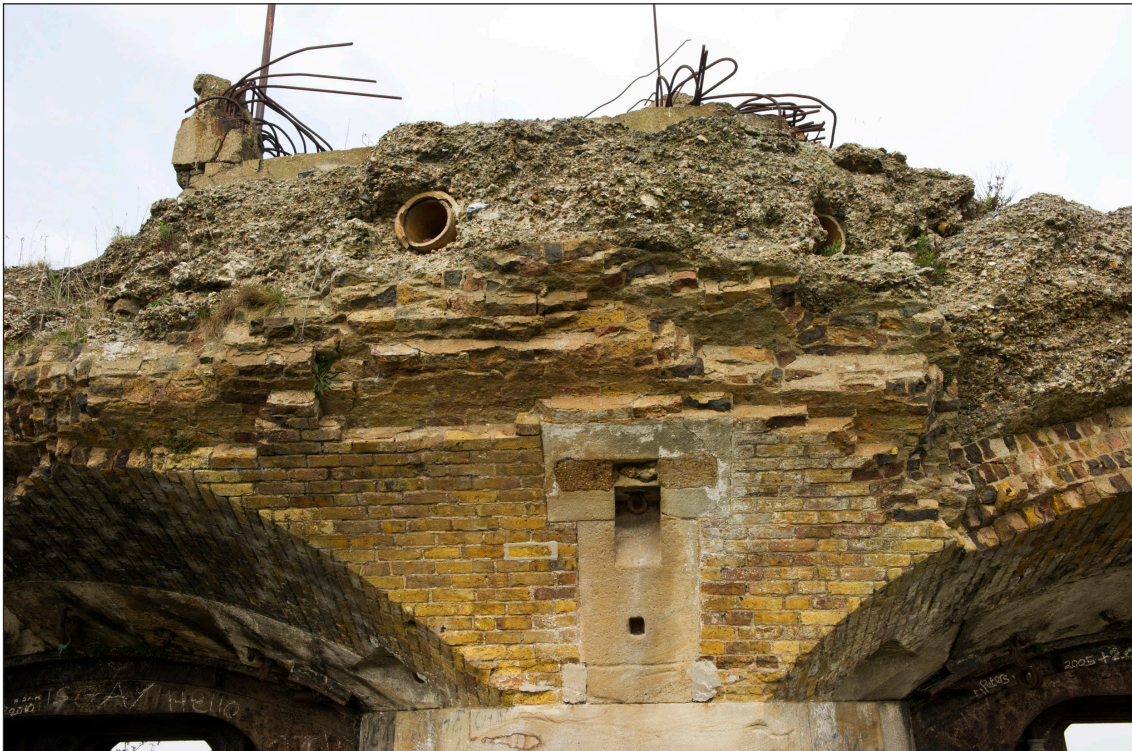
Figure 16: Detail view of the partly demolished casemated battery at Shornemead Fort. This shows the method of construction and the concrete fill used to bombproof the casemates. The earthenware ventilator pipe buried in the bombproofing and the masonry mounting for the ammunition hoist are visible. The reinforcing rods and concrete sections on the roof relate to a demolished Second World War structure. (DP097526)
