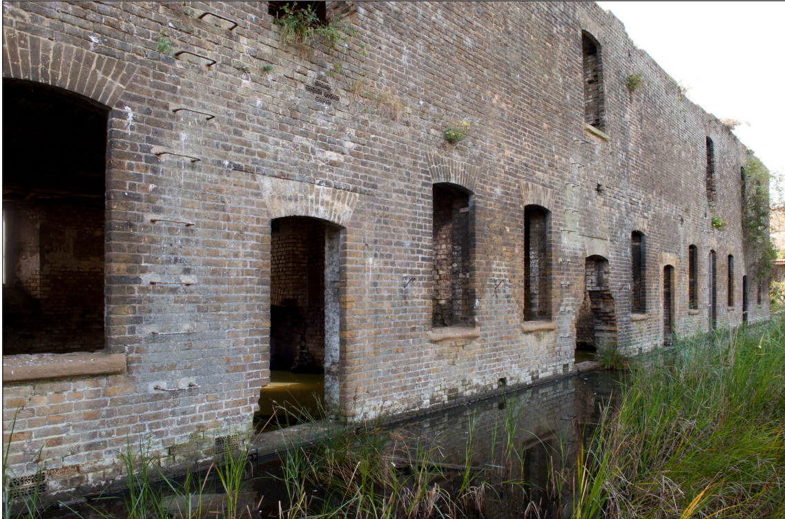
Figure 31: The north elevation of the south range showing details of the windows and doors and the iron staples of the fire escape. (DP097488)
