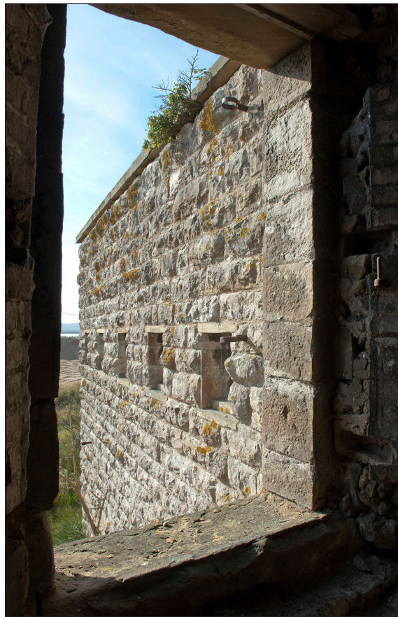
Figure 36: Loopholes on the eastern face of the south-eastern demi-bastion as seen from the hospital lavatory. Iron brackets that held downpipes can also be seen. (DP 097504)
