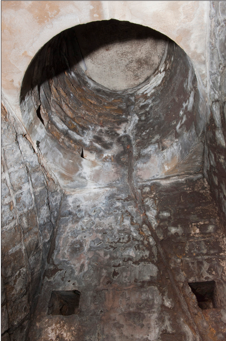
Figure 9: Detail of No 3 Shell Lift looking upwards towards the gun floor. The sockets for the collar anchors can be seen. (DP097451)
