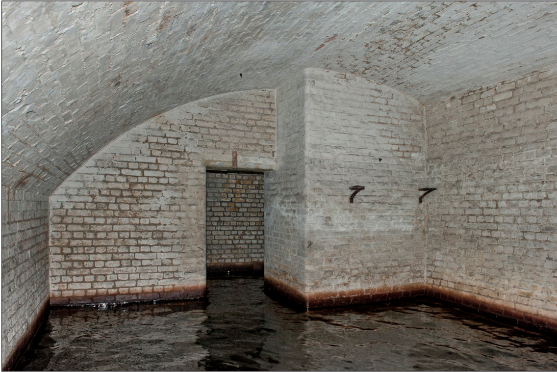
Figure 13: Interior of No 4 Cartridge Store [91] rebuilt for the insertion of a branch lighting passage. The end wall of this passage is to the right of the inserted doorway into the shifting passage. The wall brackets supported the fuse and primer box. (DP097453)
