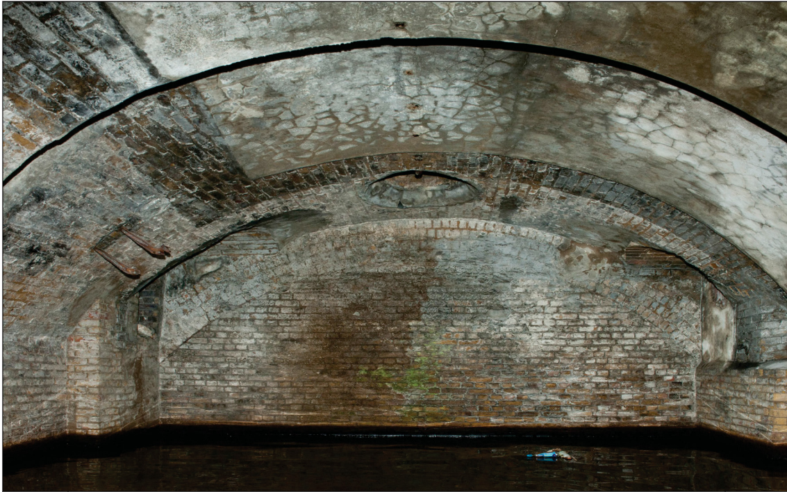
Figure 62: The interior of the former boiler room and oil store looking west. The scar of the removed wall between the ammunition store and the shifting passage is visible on the vault along with the shaft for the ammunition lift to the former open battery. The brick piers beneath the vaulted openings to the blocked shifting passage are the remains of the base and flues for the Cornish boilers. (DP 097540)
