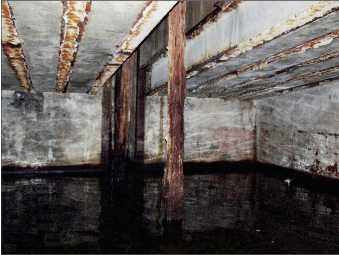
Figure 60: The interior of the Torpedo Store looking west and showing the slope of the roof to accommodate the top of the south launching slipway. The vertical timbers in the foreground mark the course of the torpedo handling slot © Wayne Cocroft
