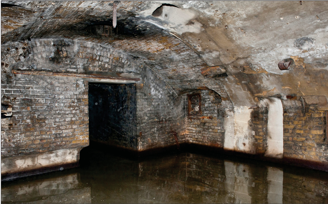
Figure 64: The interior of the Engine Room looking west. The entrance to the Torpedo Store is in the centre of the frame and to its left is the segmental head for the entrance to the caponier. In the vault, and surrounded by light coloured concrete, is the shaft pierced for the driving wire to the north slipway. The projecting iron strap is possibly a support for a pulley wheel. The deep recess at the foot of the wall on the left marks the course of the sea water supply pipes to the surface condenser. On the right the blocked arched headed opening for the shifting passage has a metal framed opening for a flue rodding point inserted in its centre. (DP097535)
