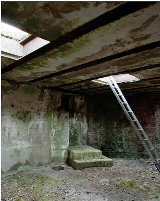
Figure 67: The opening for the north slipway pulley beam in the concrete block that occupies the embrasure of the former northern open gun position. It is located just below the ceiling with the securing studs for a pulley and the shaft leading down to the Engine Room on its left side. On their right is the short flight of concrete steps for access to the pulley beam. (DP097783)
