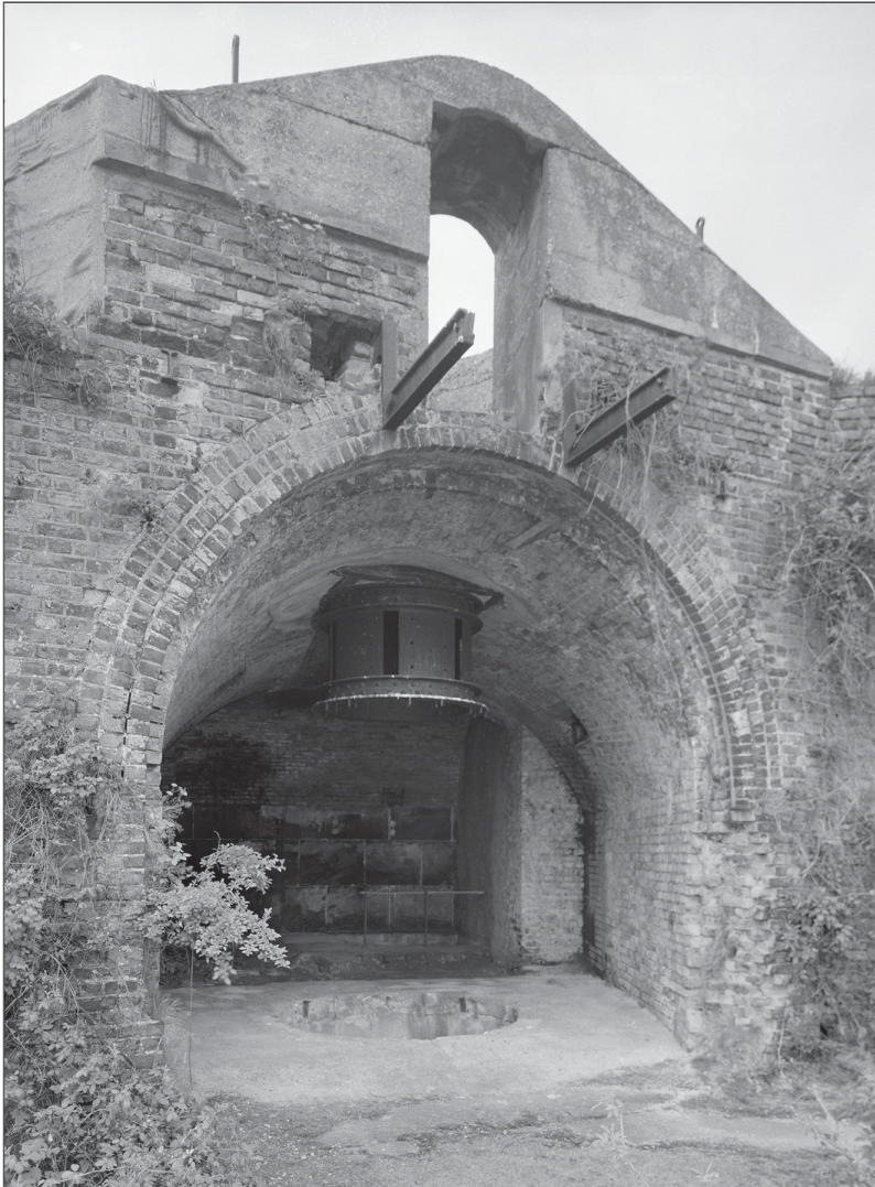
Figure 66: The gable end of what was probably the original Brennan observation position above Casemate 15. The later concrete cone for the rising tower appears to have engulfed the earlier handrail stanchions. (bb93_20789)
