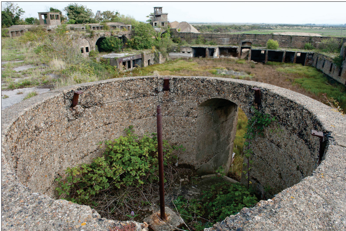
Figure 71: The interior of the collar for the rising tower looking north. The horizontal marks in the sides of the cone mark successive pours of concrete. The steeply sloped ramp between the interior of the cone and the opening in the gable end of the earlier observation position can be seen on the right hand side of the picture. The rod set in the centre is thought to be a mounting for a Second World War light machine gun sitting on an inserted timber floor. (DP097558)
