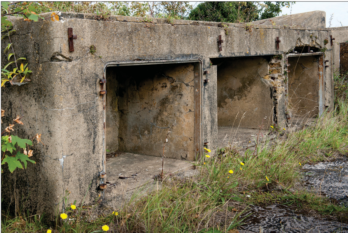
Figure 52: Ammunition lockers associated with the western 6-inch gun position. Hinges for doors on the two flanking cartridge lockers are visible as well as bolts that carried a rain hood above all three lockers. (DP097746)
