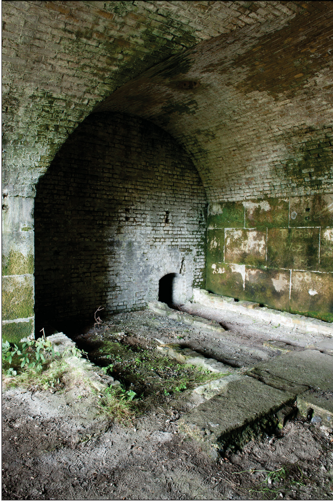
Figure 69: The southern wall of Casemate 15 showing the low tunnel that may have been inserted to enable the installation of the machinery for the rising tower. (DP097642)
