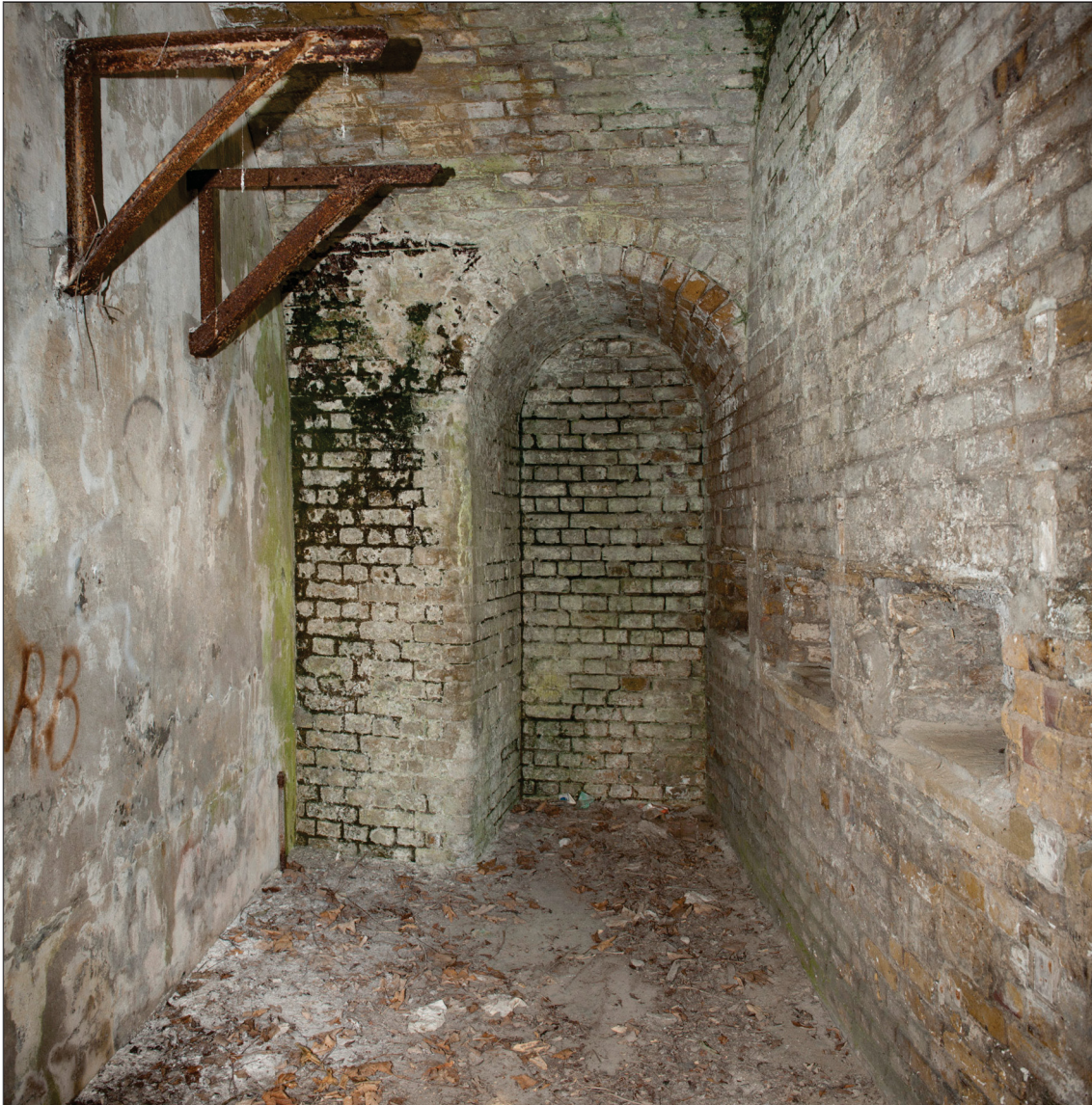
Figure 42: The south-east corner of Casemate 1. To retain access to the loopholes in the bastion wall on the right-hand side of the picture this corner of the casemate was not filled with concrete when the rest of the position was converted to a traverse. The smooth concrete wall of the traverse is on the left-hand side (the brackets are later additions). (DP097610)
