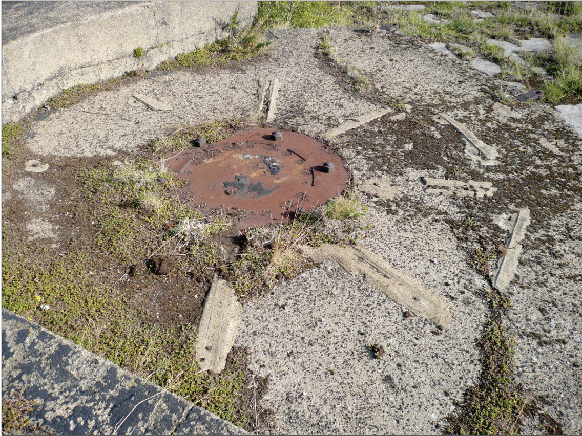
Figure 57: Most southerly 12-pounder emplacement with possible evidence of adaptation at a later date. (DP097777)
