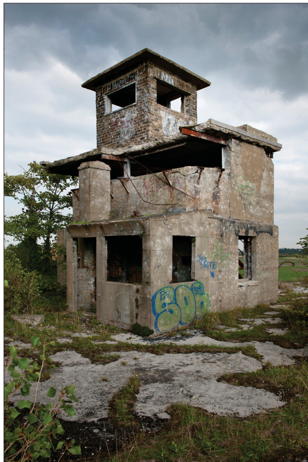
Figure 53: The Battery Observation Position looking east. The chimney stack of the projecting single-storey structure obscures the view from the observation slits. The hut on the roof dates from the Second World War. (DP097671)
