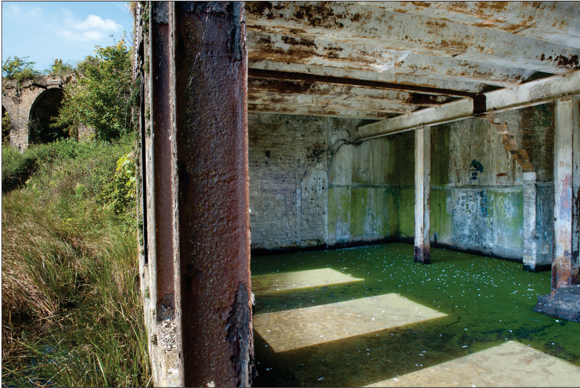
Figure 73: The interior of the Engine and Dynamo House [70, 71]. The later (presumed Second World War) steel-beam and ribbed-section roof can be clearly seen. The black stripe running across the roof indicates the position of the former dividing wall between the Engine and Dynamo Rooms. The corner of the engine base can just be seen to the right of the picture. (DP 097558)
