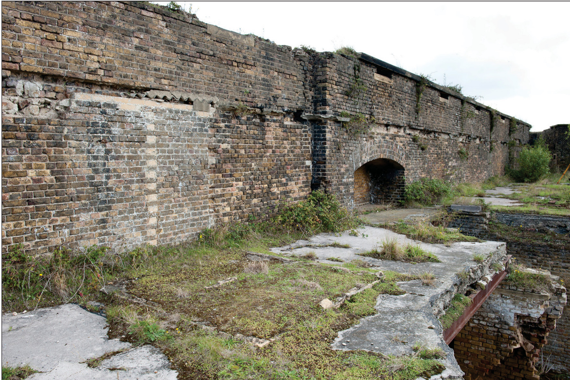
Figure 77: Former position of the possible signals hut on the roof of the entrance range. (DP097582)
