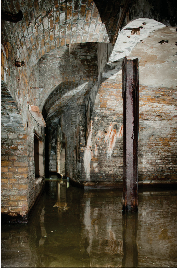
Figure 68: The former lighting passage running at the rear of the Brennan Installation. The Engine Room is in the vaulted casemate to the right with the later condenser tank and pumps in the adjacent casemate, the entrance to which is just visible at the end of the passage. The rectangular recess visible in the wall on the left side may be connected with the support for the engine steering beam. The manhole that opens into the former open gun emplacement above is in the cut out section of the lighting passage vault. (DP 097528)
