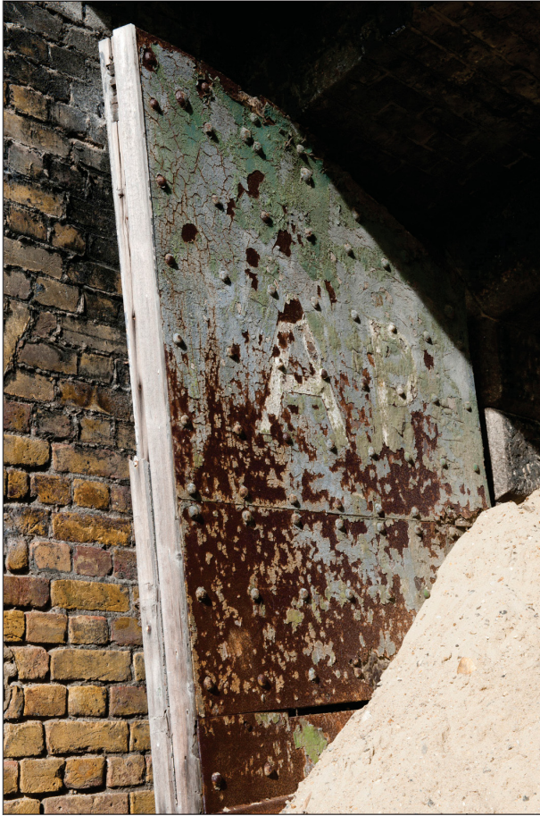
Figure 78: The right-hand leaf of the front doors to the fort. Evidence for the occupation of the fort by the Royal Naval Auxiliary Patrol is provided by the letters 'A P' on a background of flaking naval grey paint. (DP097676)
