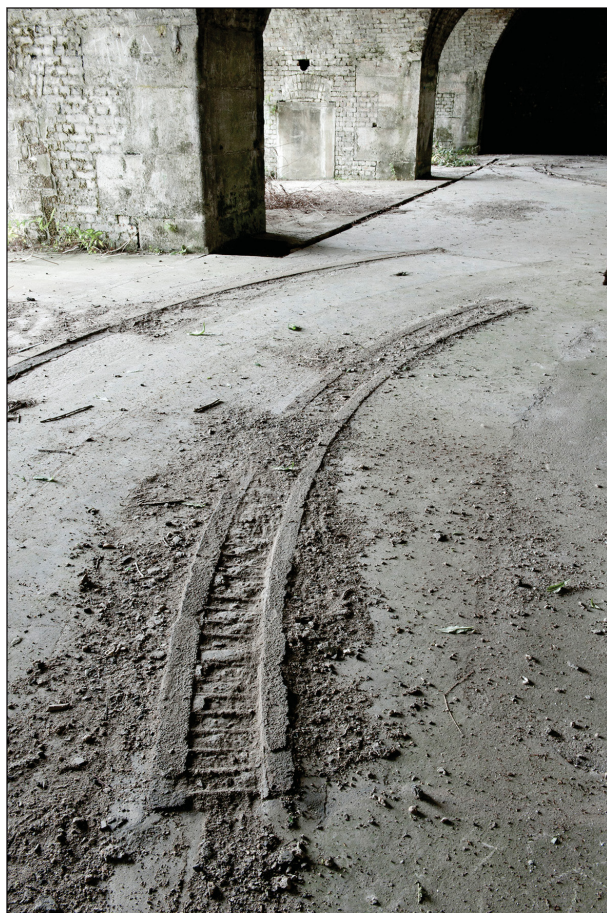
Figure 43: The cogged racer rail in Casemate 12 suggesting that alterations were made to the carriages in this casemate. (DP097629)
