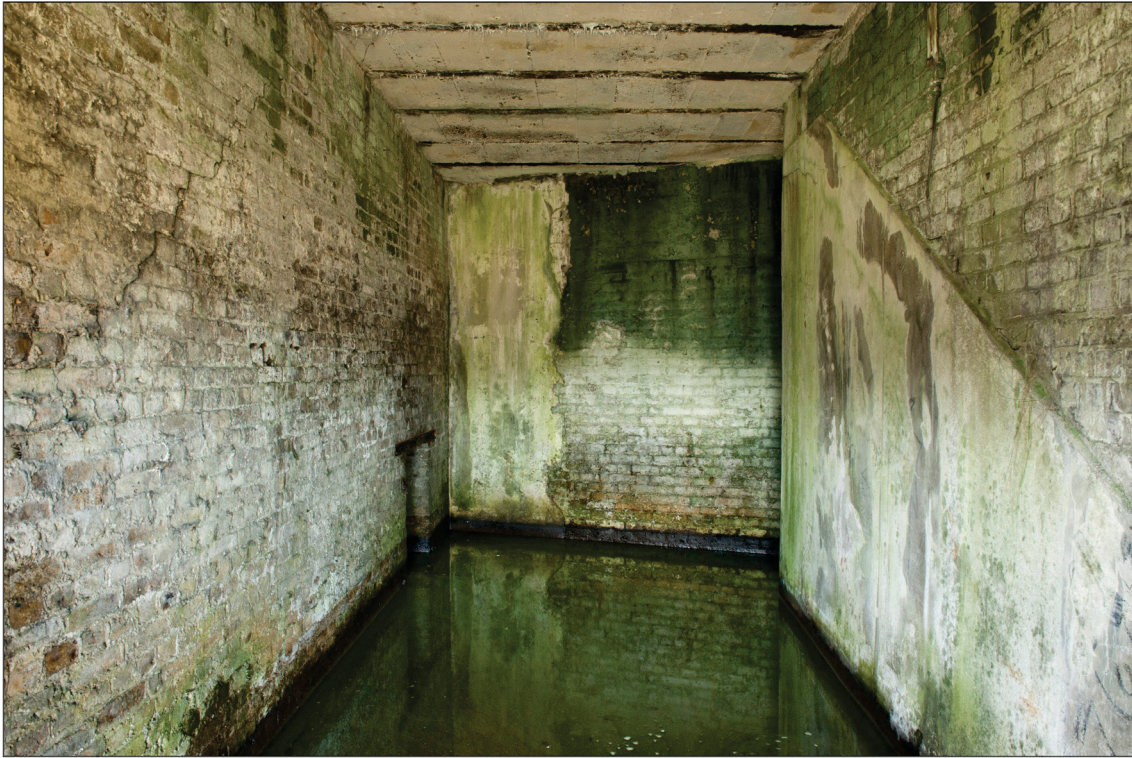
Figure 63: The interior of the coal store with the coal hatch at the base of the left hand wall and the render on the right hand wall marking the line of the original traverse. (DP097545)
