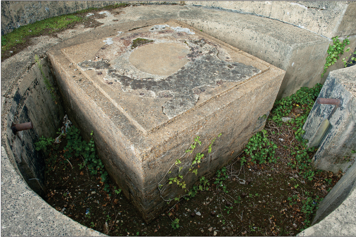
Figure 79: Concrete block inserted to modify the 6-inch gun emplacements during the Second World War. (DP097671)
