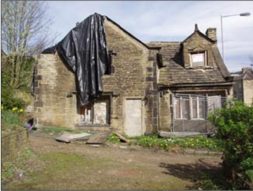
Fig 9: south elevation, with cross wing to left and housebody to right (© English Heritage)
