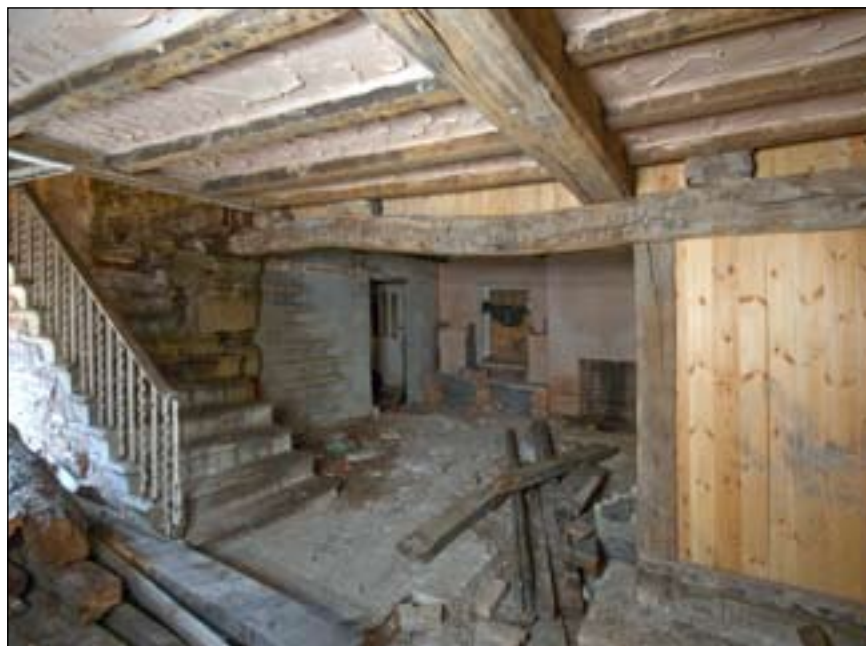
Fig 23: west wing, view to north-east showing inserted stone stair with iron balusters (DP071458 © English Heritage)
