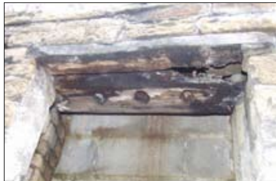
Fig 15: lintel of timber-mullioned window, west cross wing, west wall north end (© English Heritage)
