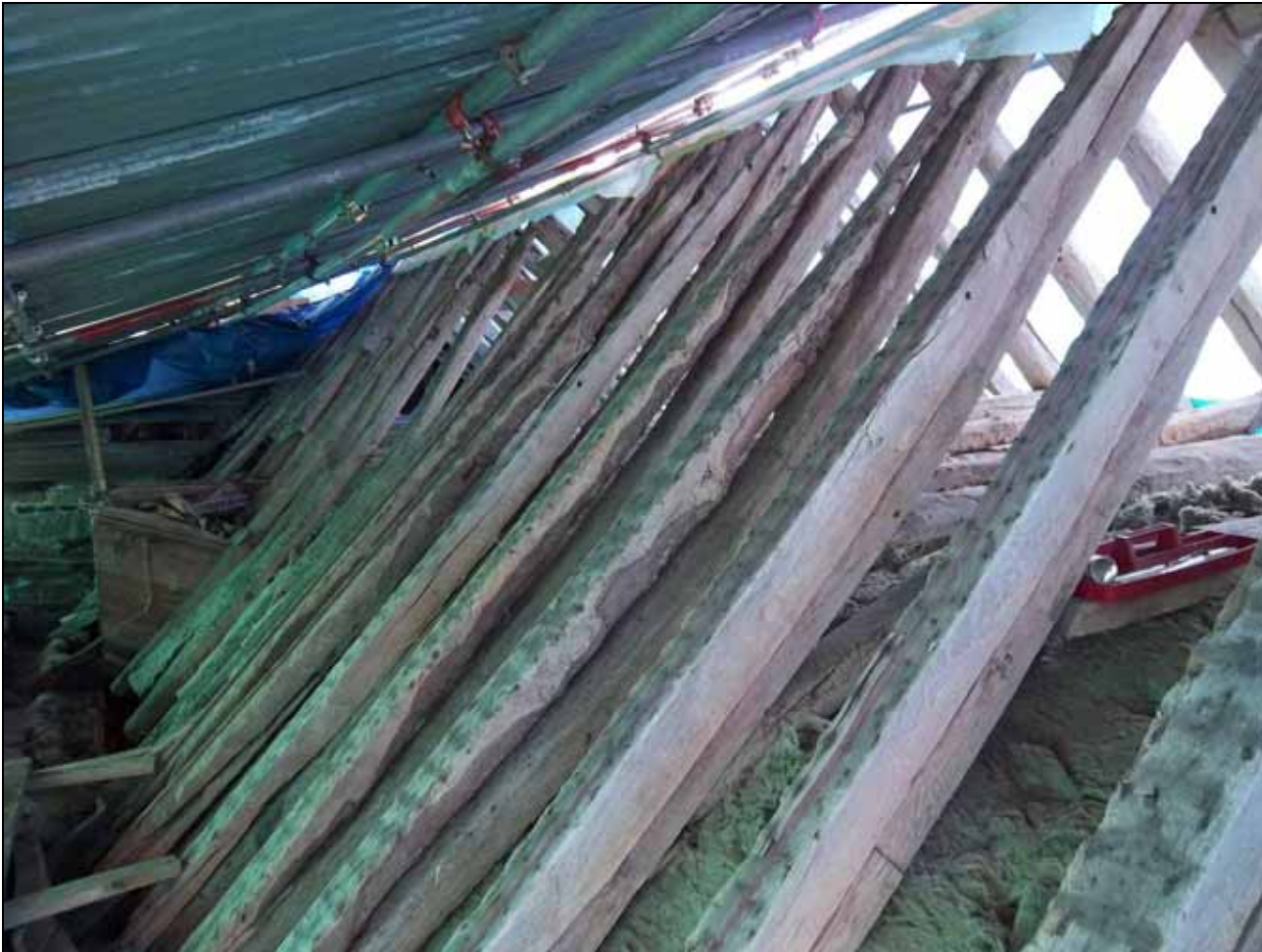
Figure 4: Nave roof showing the backing rafters (photograph taken from the south-east). Photograph Robert Howard
