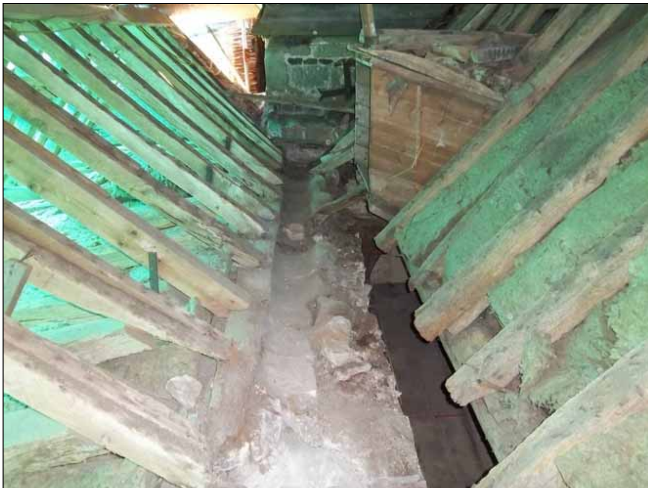
Figure 7: Stone gully between south aisle (to left) and nave (to right) roofs. Photograph Robert Howard
