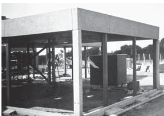
Figure 4.28: Ernehale Primary School, Arnold, under construction in 1969. Reproduced by kind permission of Nottinghamshire Archives.
