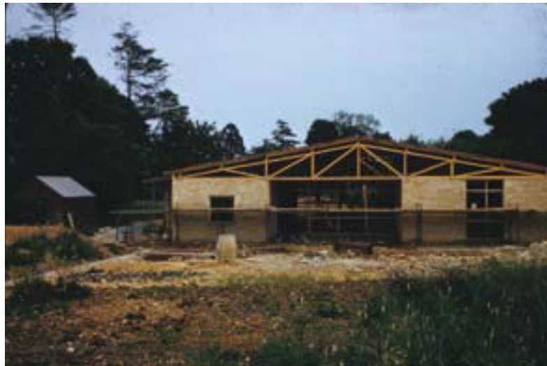
Figure 3.5: 'Rat. trad.' construction at Finmere Primary School, Oxfordshire in 1959. Lightweight, exposed timber trusses rests on load-bearing panels of brickwork; the timber-framed window-walling is last to be installed. For the plan of this school see fig. 2.4. Institute of Education Archives: ME/Z/5/2/150.
