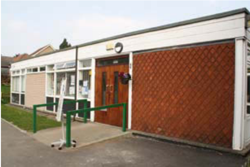
Figure 4.41: Tiling hanging at the CLASP Orchard Infant School, Sprotbrough, Doncaster; Twist & Whitley, completed 1966. Ken Twist and Ken Evans worked together at the Hertfordshire Architect's Department in the early 1950s (P5925004).
