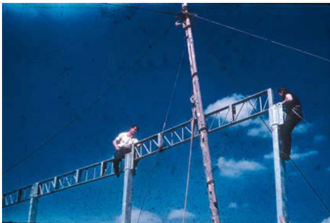
Figure 3.1: Erecting the steel frame at St Crispin's Secondary Modern School, Wokingham, built to the Hills system in 1951-53. Institute of Education Archives: ABB/B/1/75/1.
