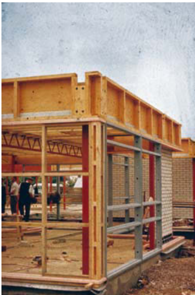
Figure 3.6: Yatton Junior School, Somerset in construction c.1967. The Consortium for Method Building employed a wide range of materials and components, some prefabricated, others assembled on site. Institute of Education Archives: ABB/B/9/14/1
