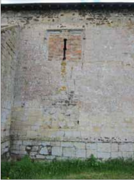
Figure 23. Blocked window at upper level with surviving hood mould on east façade.
