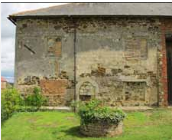
Figure 5. Blocked features on west façade.
