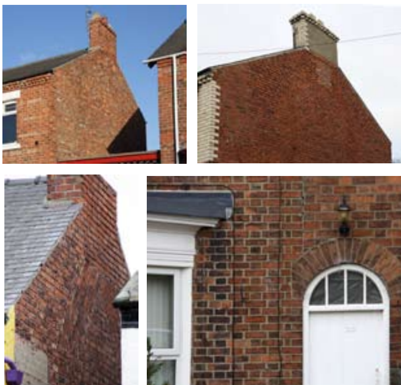
Figure 56 (top left) an externally expressed flue at No. 51 Milton Street (P5924030); 57 (top right) and at No. 27 Cobden Street (P5924031); 58 (bottom left) and at No. 172 Yarm Road (P5924032); 59 (bottom right) an example of an erratic party wall at No. 116-118 Eastbourne Road (P5924033)
