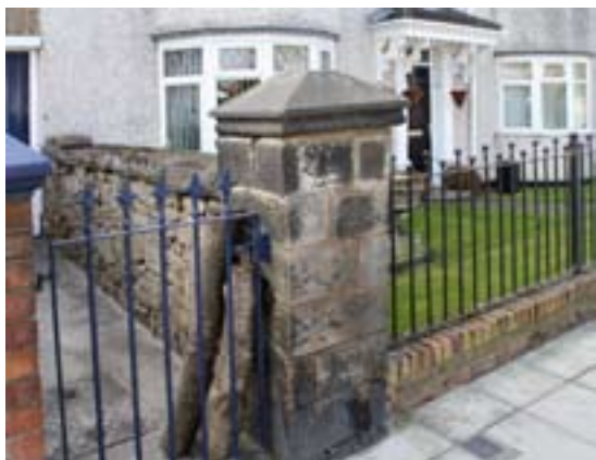
Figure 60 Stone blocks and rubble construction in the pier and front wall of No. 142 Yarm Road (P5924034)
