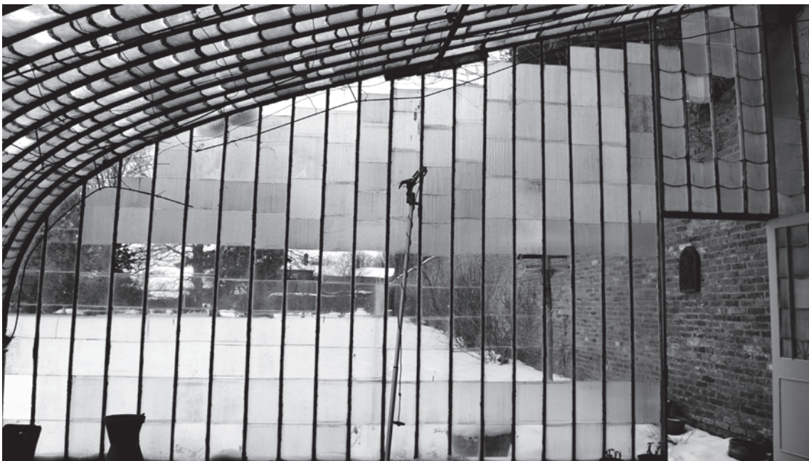
Figure 2. The west end of the greenhouse, comprising of an iron door complete with fish scale glazing. This can also be seen in the panel about the door. The glass in this end wall varies in thickness and chemical composition, and hence manufacturing dates.
