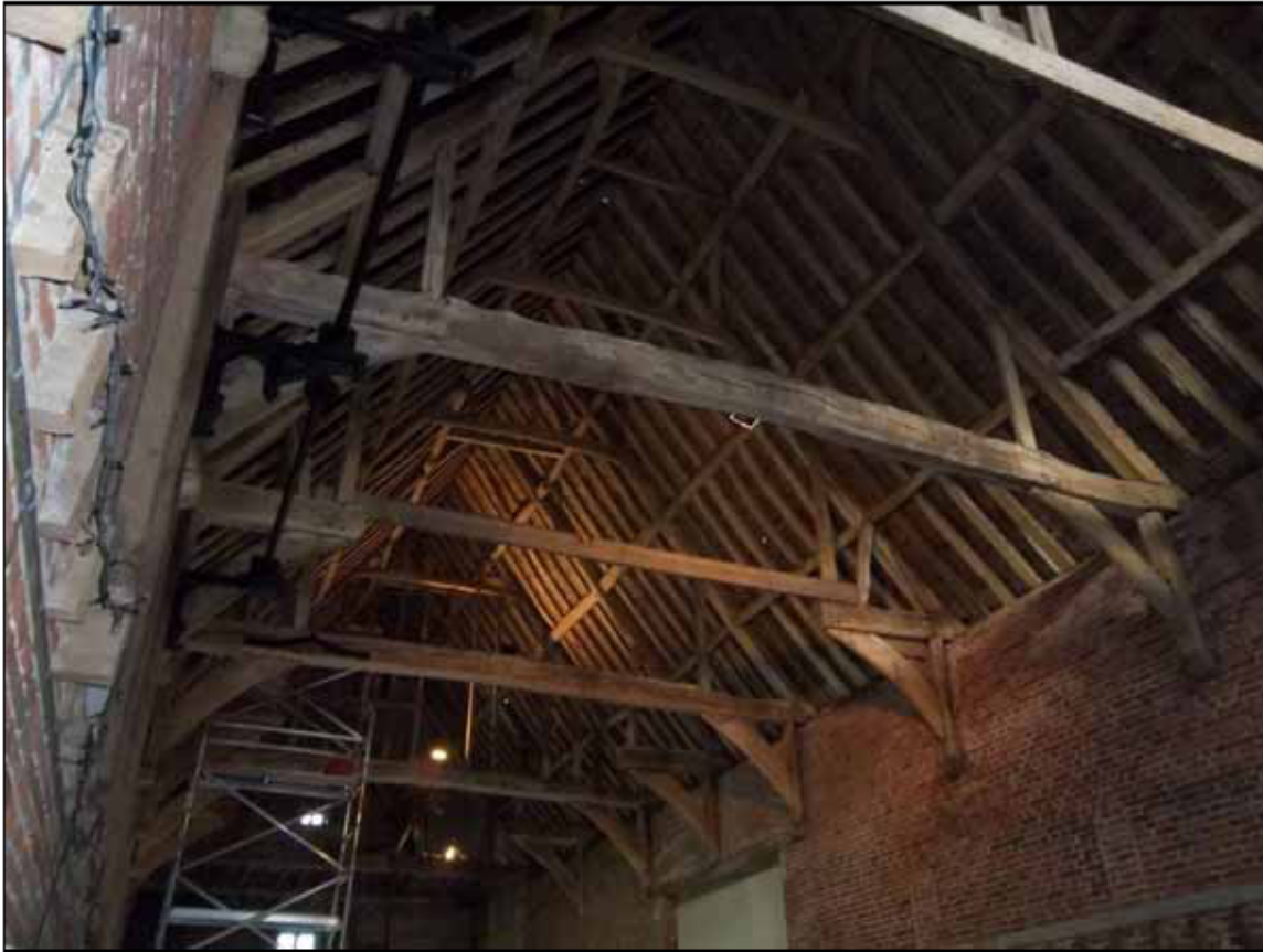
Figure 3: Godwick Great Barn roof (photograph taken from the south-west) Photograph Robert Howard
