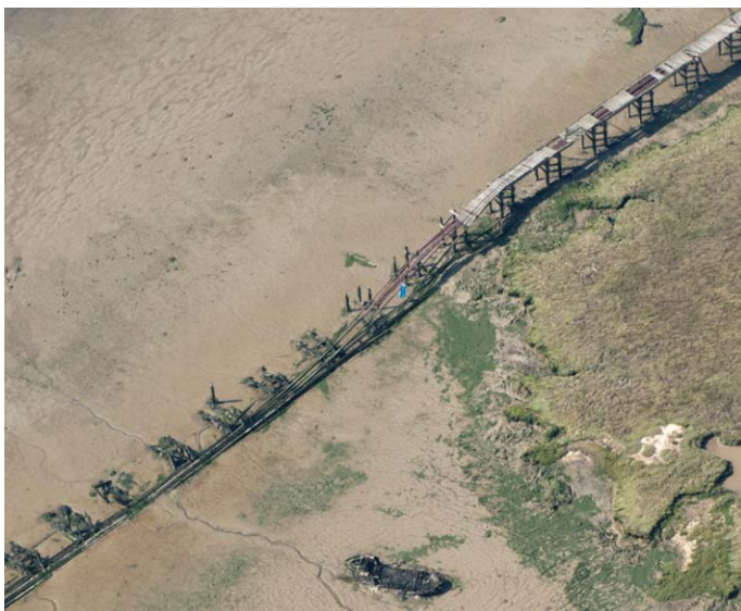
Figure 9 Collapsed section of Bees Ness Jetty. Detail of 27196/023 31-Aug-2011 © English Heritage.
