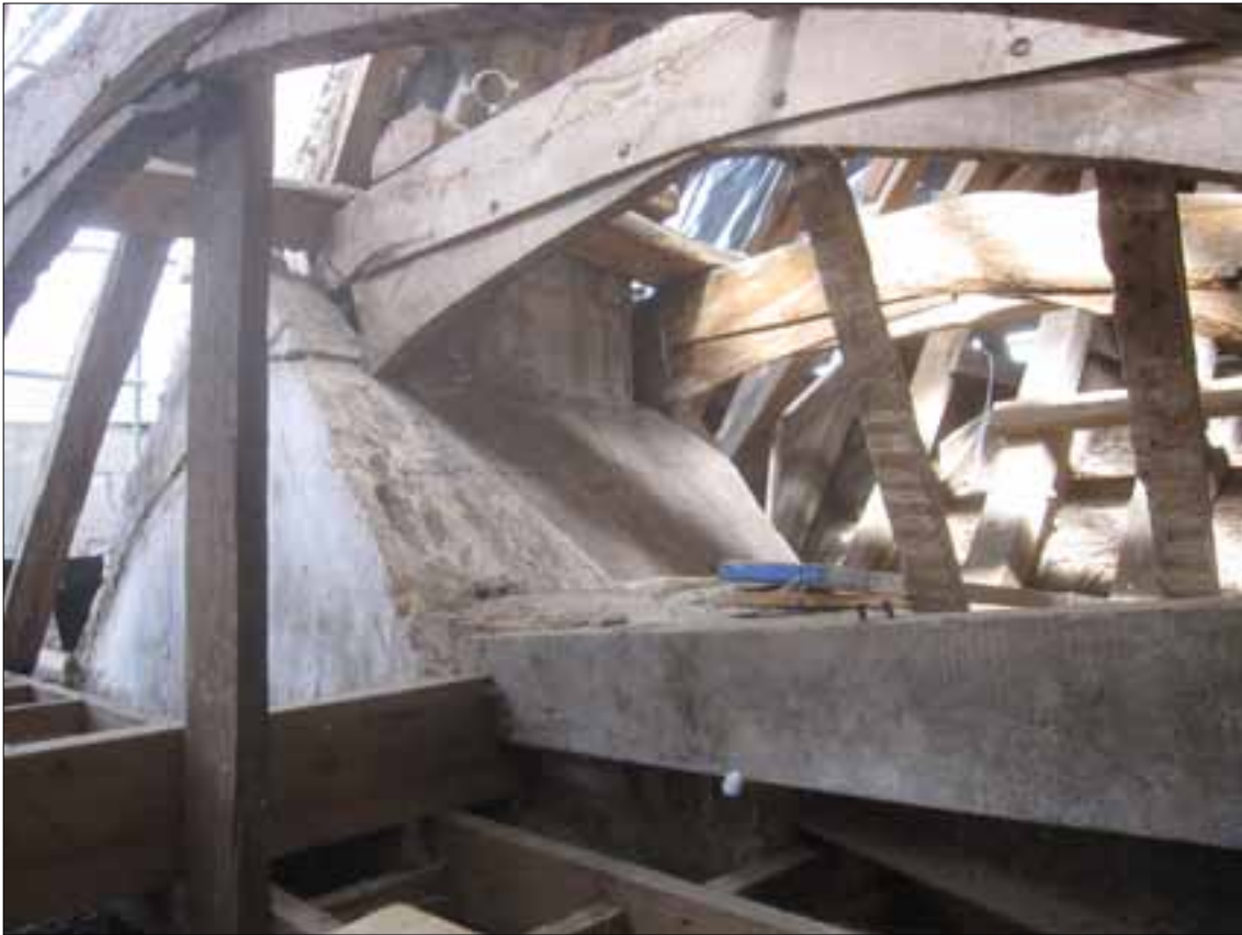
Fig 5.7 Truss T2 with south end cut off by inserted chimneystack, and canted joists to support the end of the vaulted ceiling (Nick Hill).
