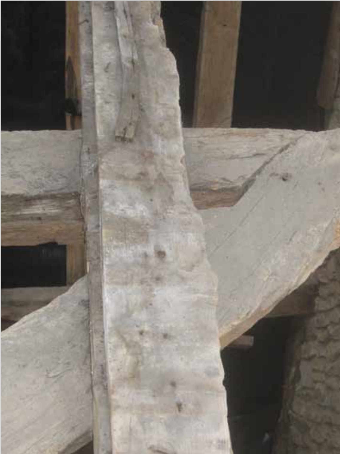
Fig 5.20 Detail of wind-brace to west section of roof, with original lapped and nailed joint to purlin (Nick Hill).
