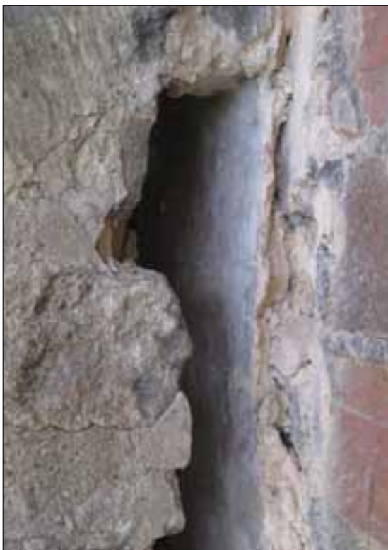
Fig 2.3 Plaster finish to north range, trapped by addition of western section of garderobe block (to left) (Nick Hill).
