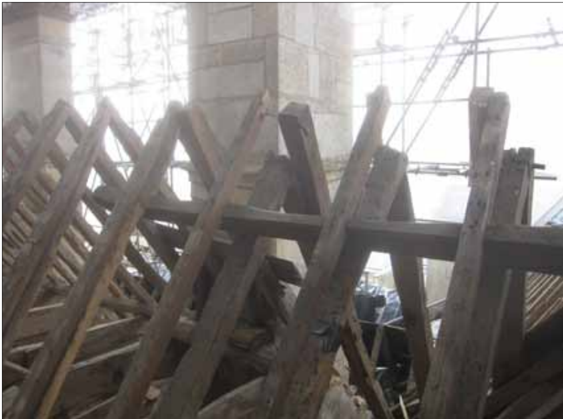
Fig 5.9 The three rafter couples at the east end of the roof which are off-set and lower than the rest of the structure (Nick Hill).
