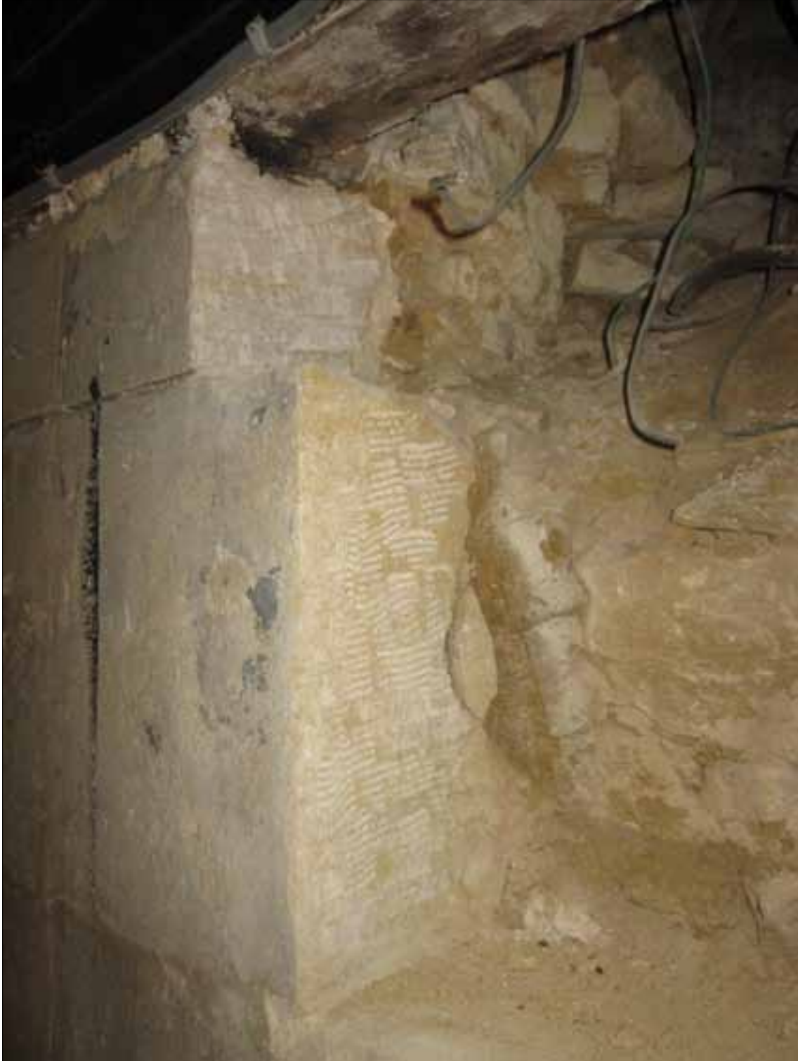
Fig 3.2 Detail of stone ashlar lining, which is well bonded and integral to the 15th-century wall structure of the Gatehouse (Nick Hill).
