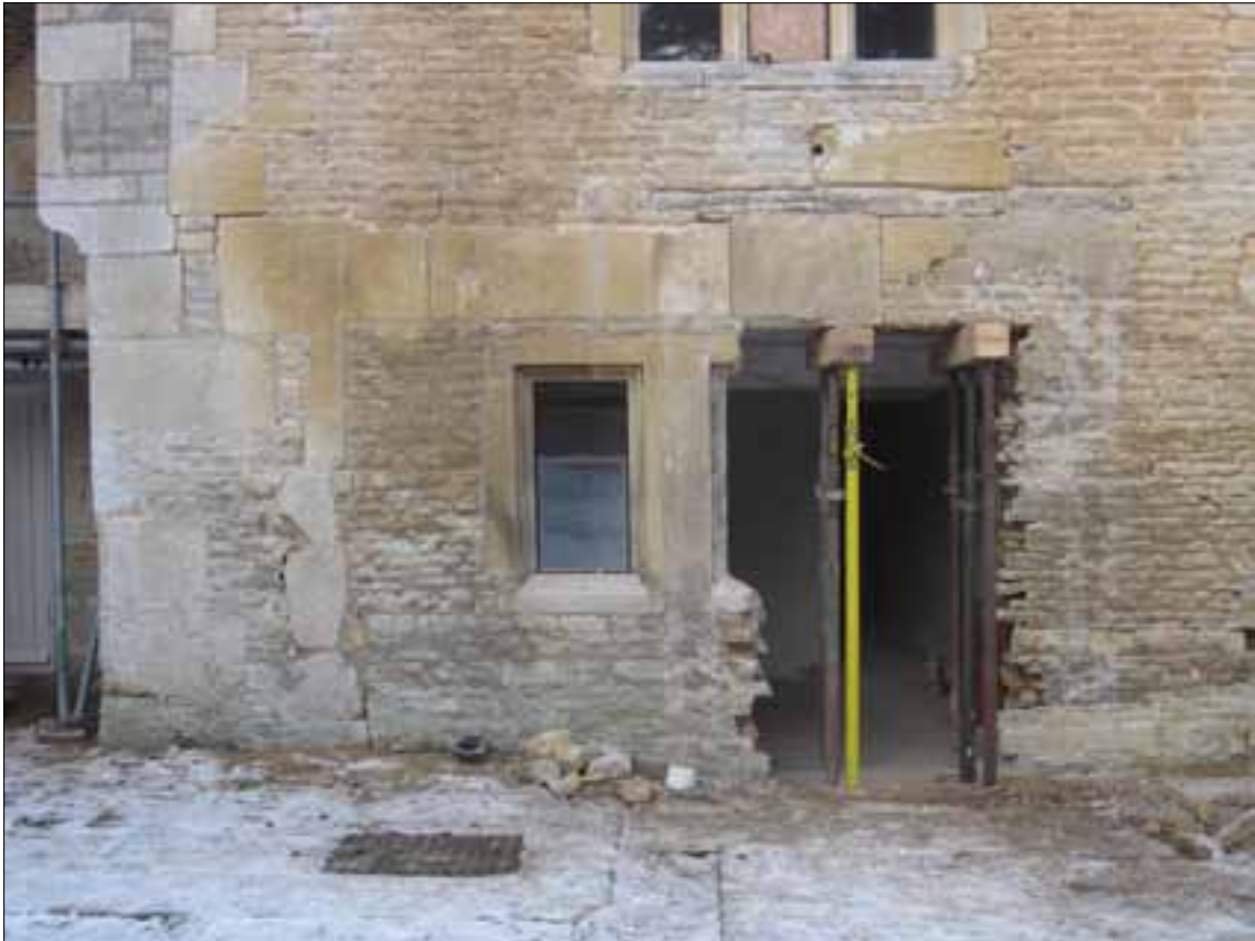
Fig 4.2 Opening up of north wall of Kitchen Court, where modern window was inserted in place of mid-20th-century doorway (Nick Hill).
