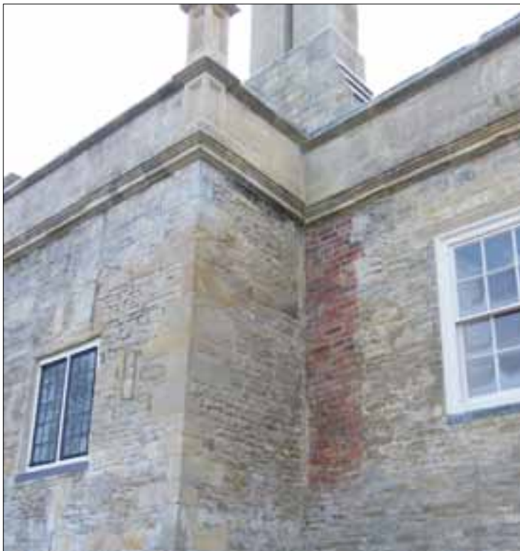
Fig 2.1 Junction of garderobe block with north wall of north range (Nick Hill).
