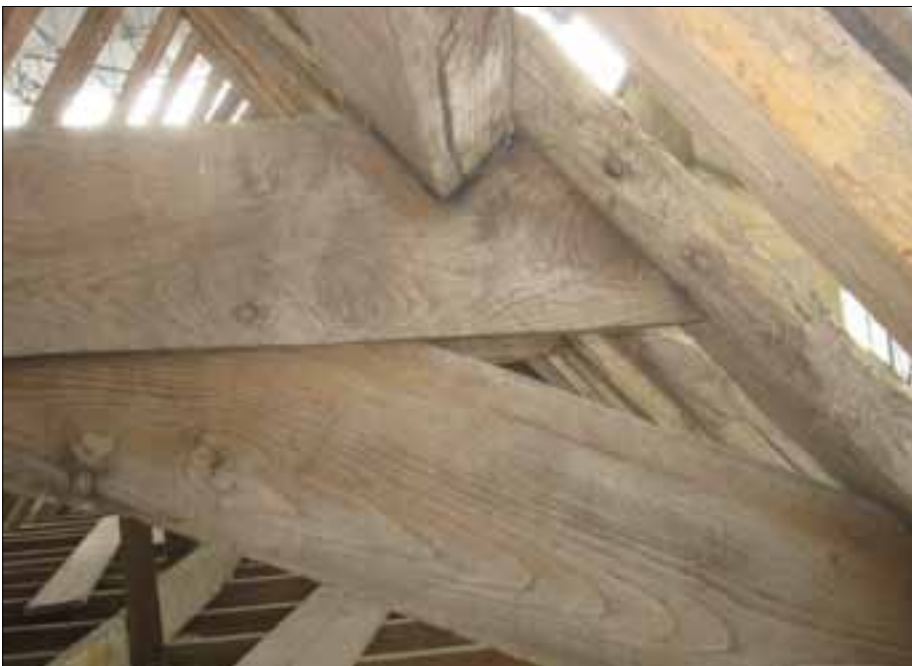
Fig 5.16 Detail of clasped purlin joint to east section of roof. Note the setting-out line and filler block for enlarged cut-out to receive purlin (Nick Hill).
