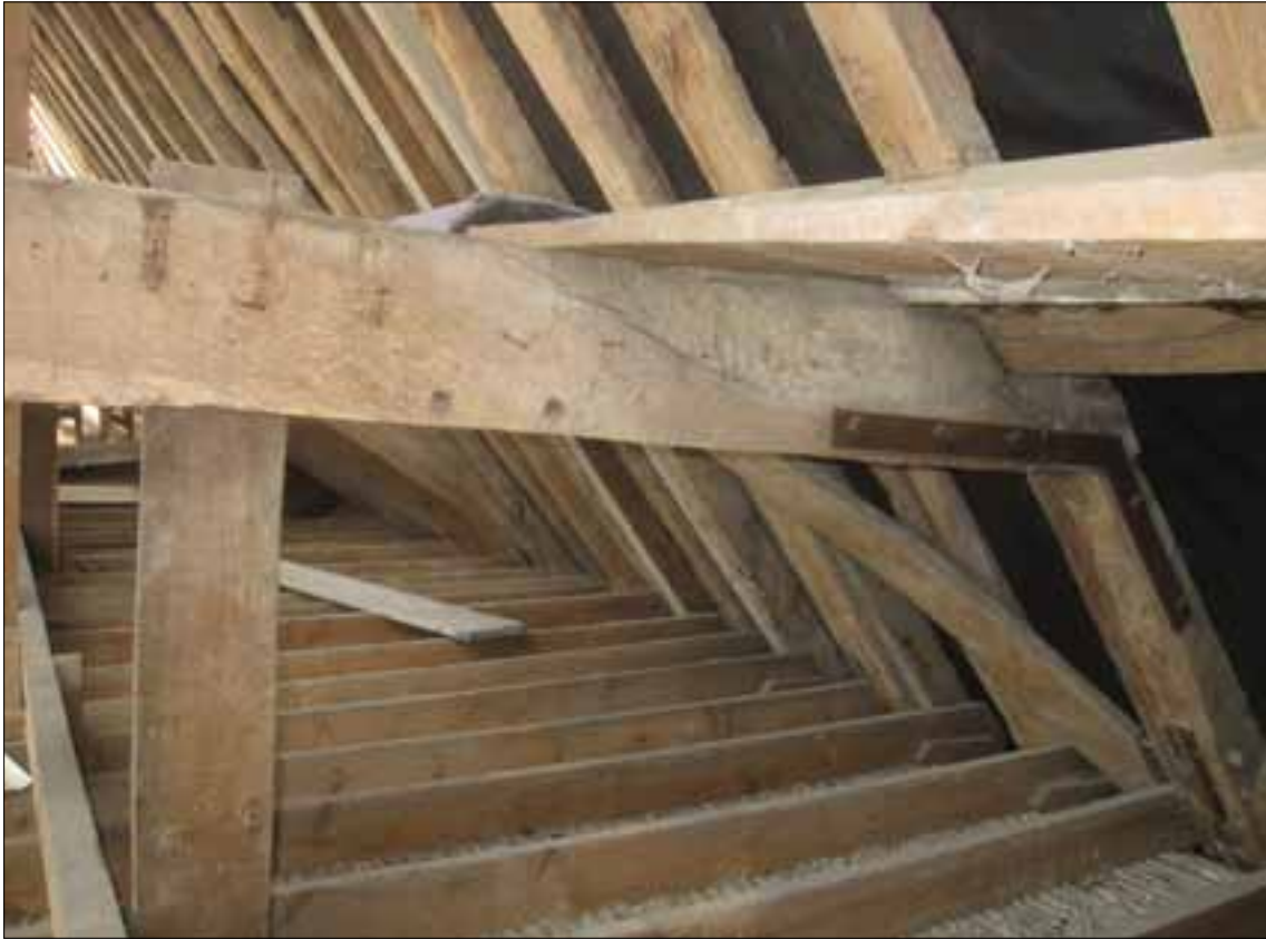
Fig 5.18 Truss T10 of west section, west face – note missing arch-brace (Nick Hill).
