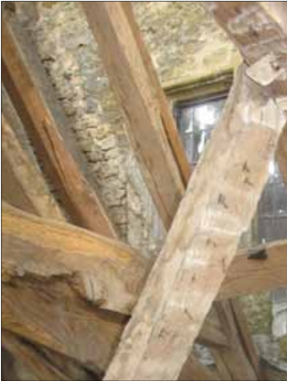
Fig 5.8 Detail of canted joists to support the end of the vaulted ceiling (Nick Hill).
