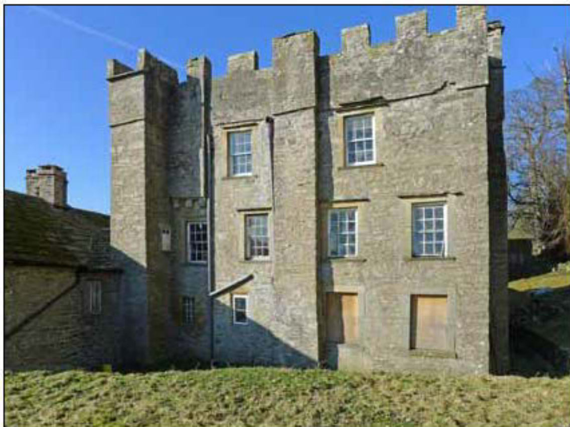
Figure 7. The east elevation of the low-end tower (photograph: Lucy Jessop, English Heritage)
