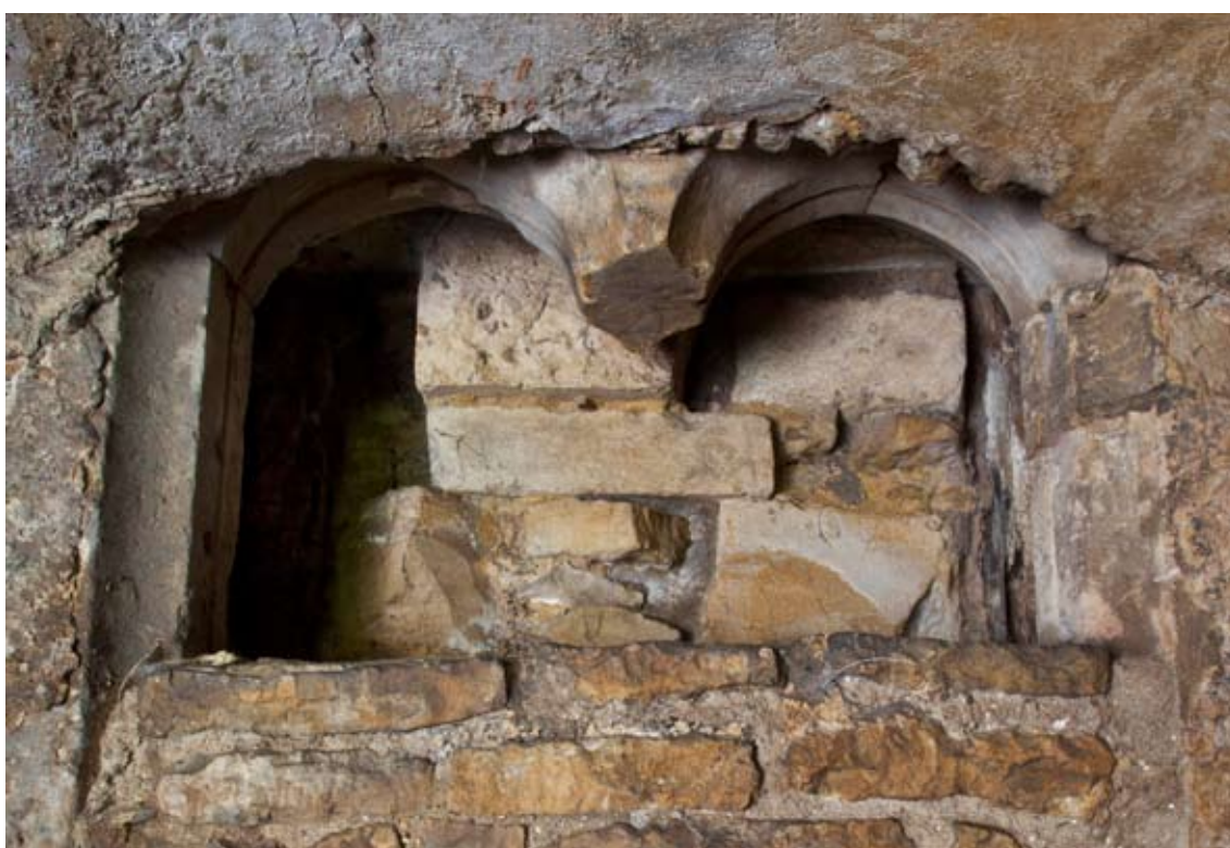
Figure 18: The two-light window partially concealed in the north wall of the stair tower
